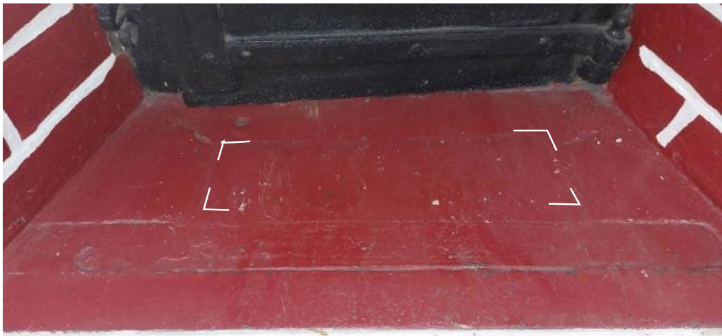
Figure 42 The cill of the oven opening showing the blocked opening (the corners of which are marked) where ash raked from the oven would fall to the ash pit below. In front of this opening is an iron clamp.
