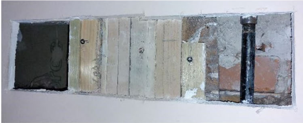
Figure 50 Modern stud infill to the former wide opening between the current master bedroom and bathroom with the original brick reveal to the right.
