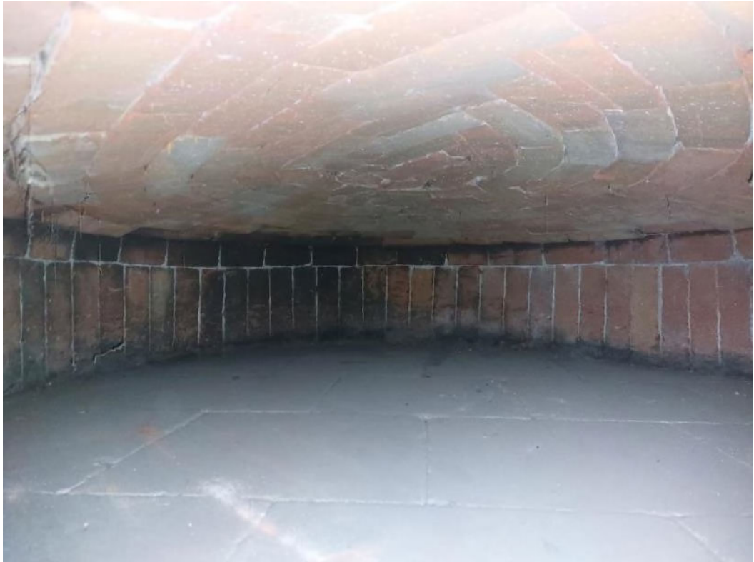
Figure 46 Interior of the oven chamber.
