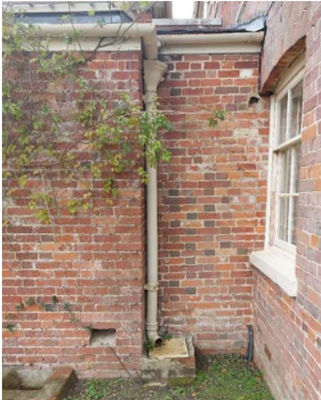
Figure 26 The short section of brickwork which is recessed so that the south-west wall of the oven building avoids the adjacent window to the right. The quality of this brickwork is lower than that of the main block of the oven building.
