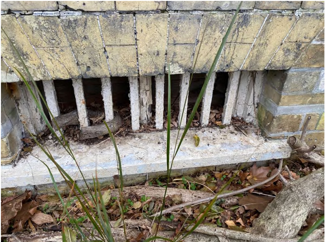
Figure 54 External side of the opening to the cellar room where the extractor will vent – the vent will be set behind the bars and will not be visible externally.
