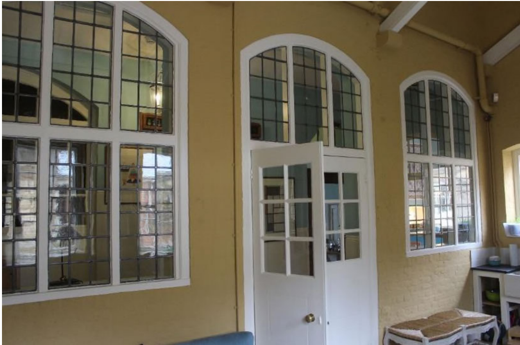
Figure 36 Webb's windows and double doors between the service passage and the former covered yard.
