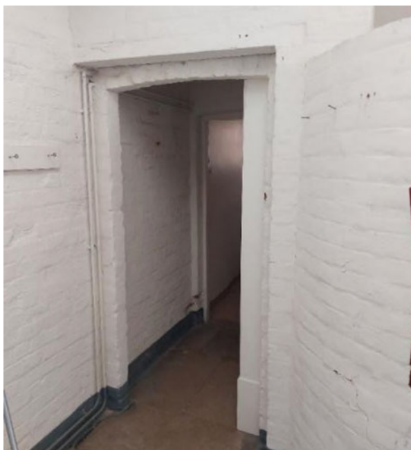
Figure 39 The opening from the oven room to the WC showing the square-headed opening with a segmental arch to the second skin of brickwork, the same arrangement used for the second door to the WC which can be seen in the background.
