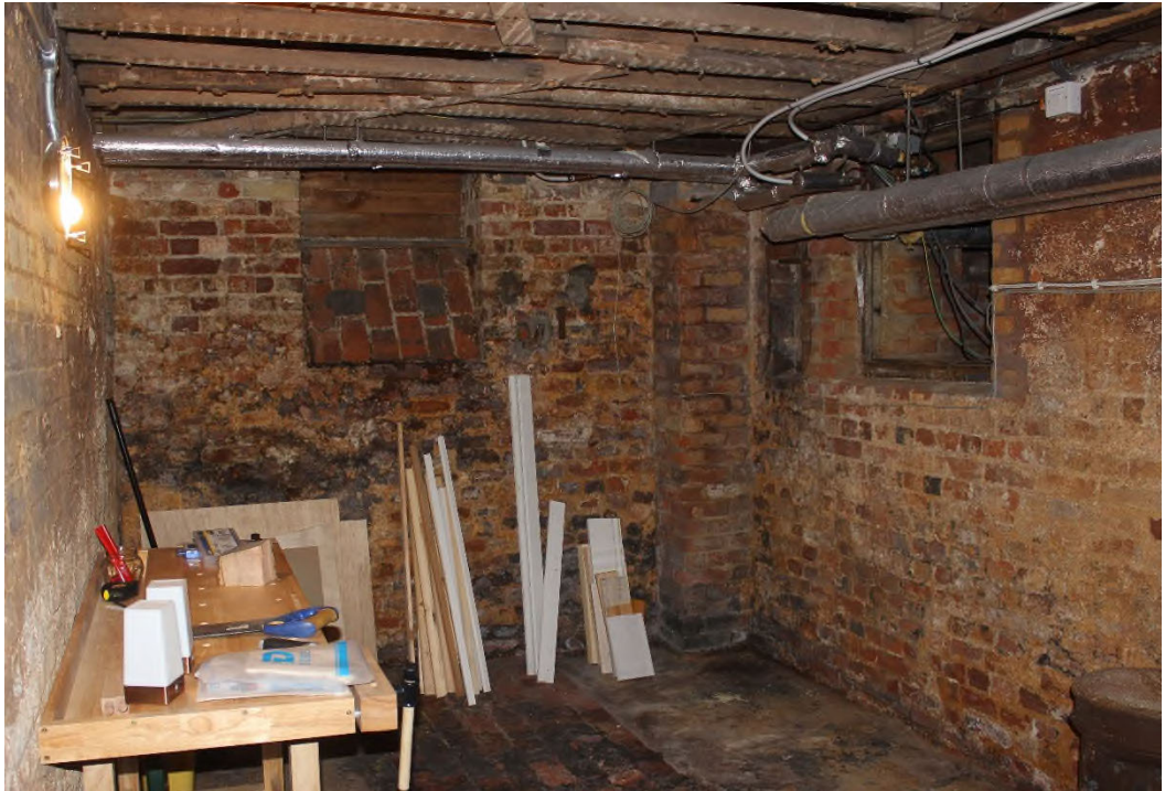
Figure 53 The cellar room adjacent to the floor void of the common room showing the opening to the floor void to the right and the opening where the extractor will vent to the left with the sloping brick cill.
