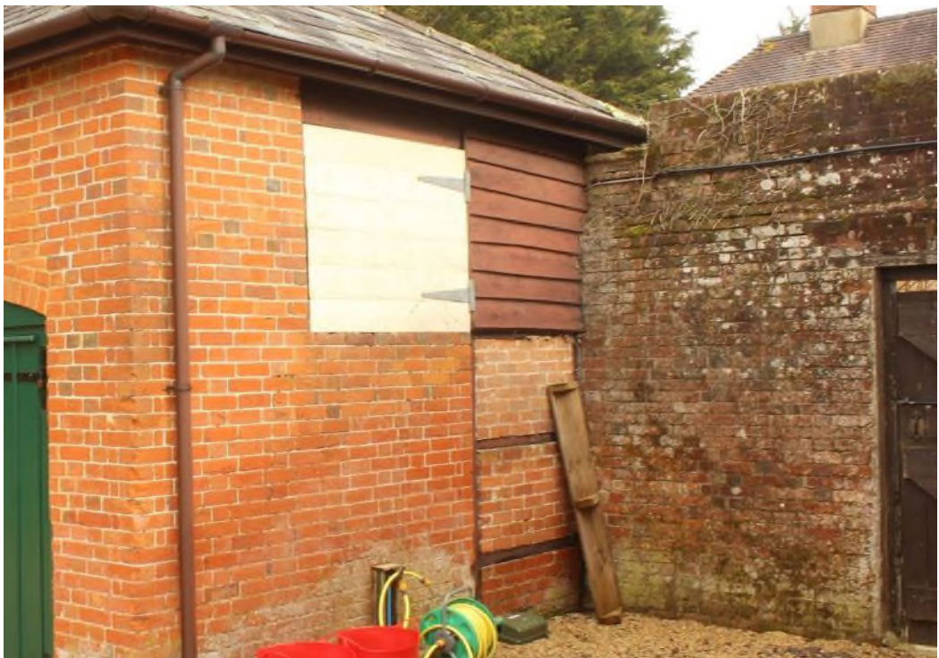
Figure 56 The section of wall between the slaughterhouse and stables on the south-west side of the kitchen garden showing the simple step down in the wall height to respect the eaves of the slaughterhouse.
