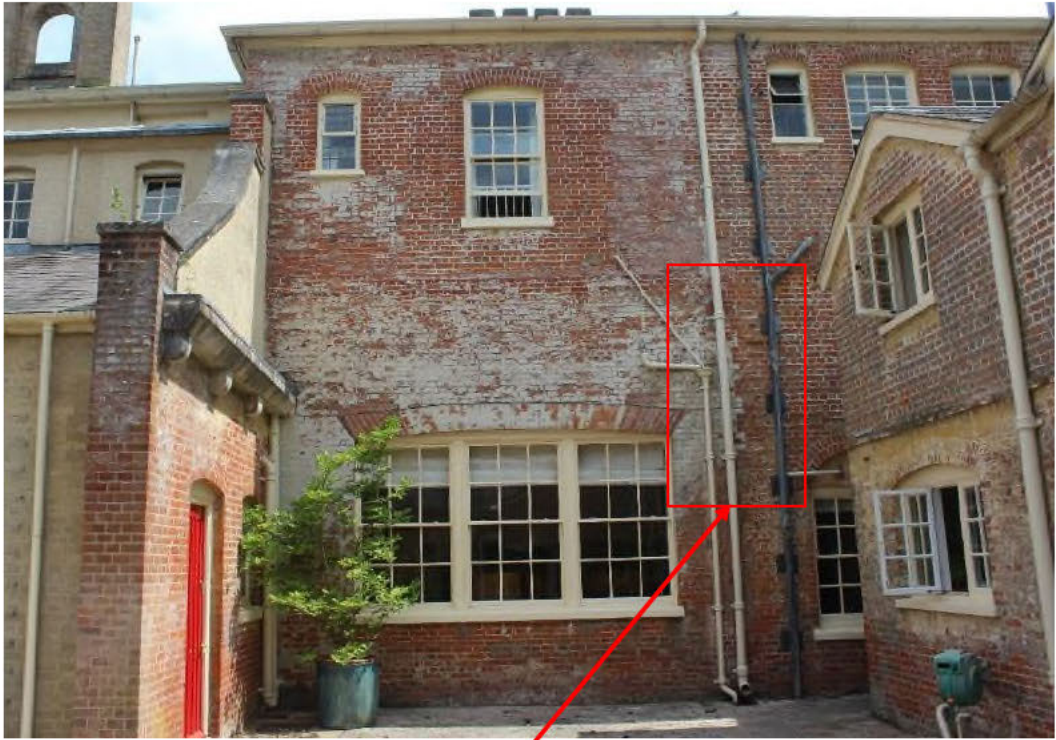
Figure 21 North-west elevation of the service range with a detail showing the keyed junction between the two phases of construction.
