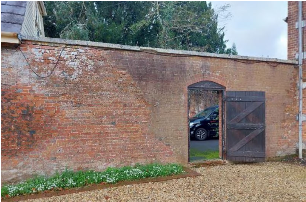
Figure 28 The wall between the estate office and the service range, south-east side.
