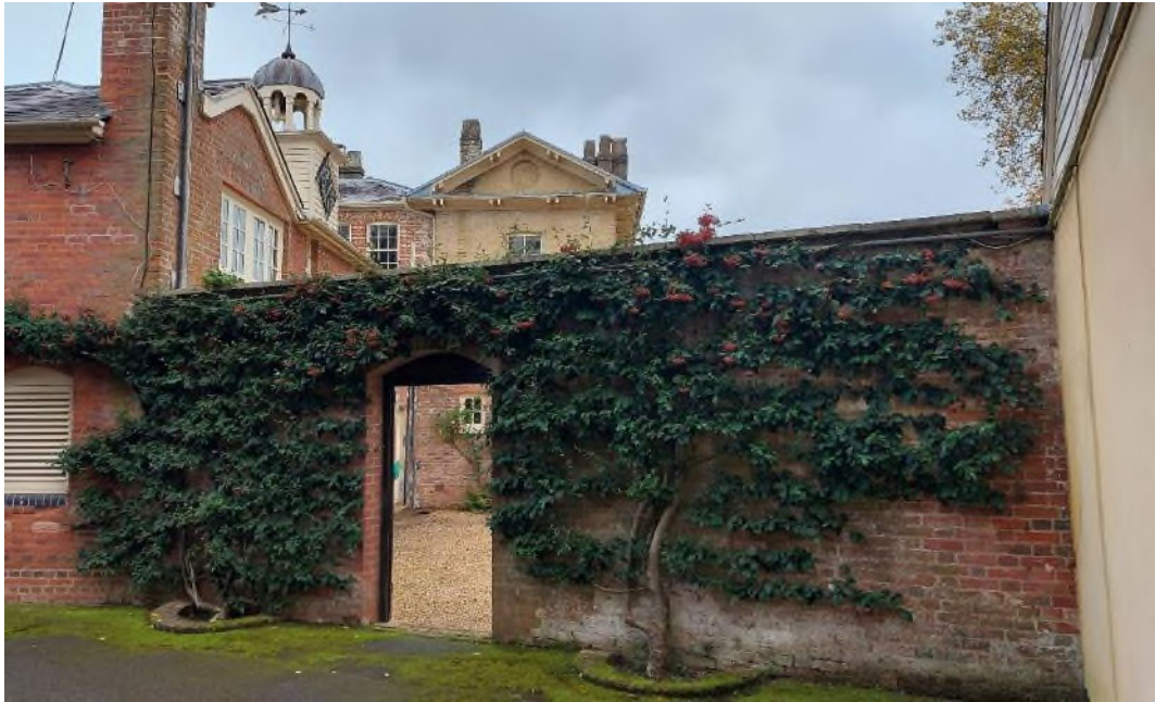
Figure 57 The wall closing the gap between the service wing (left) and the estate office (right) from the yard area adjacent to the estate office.
