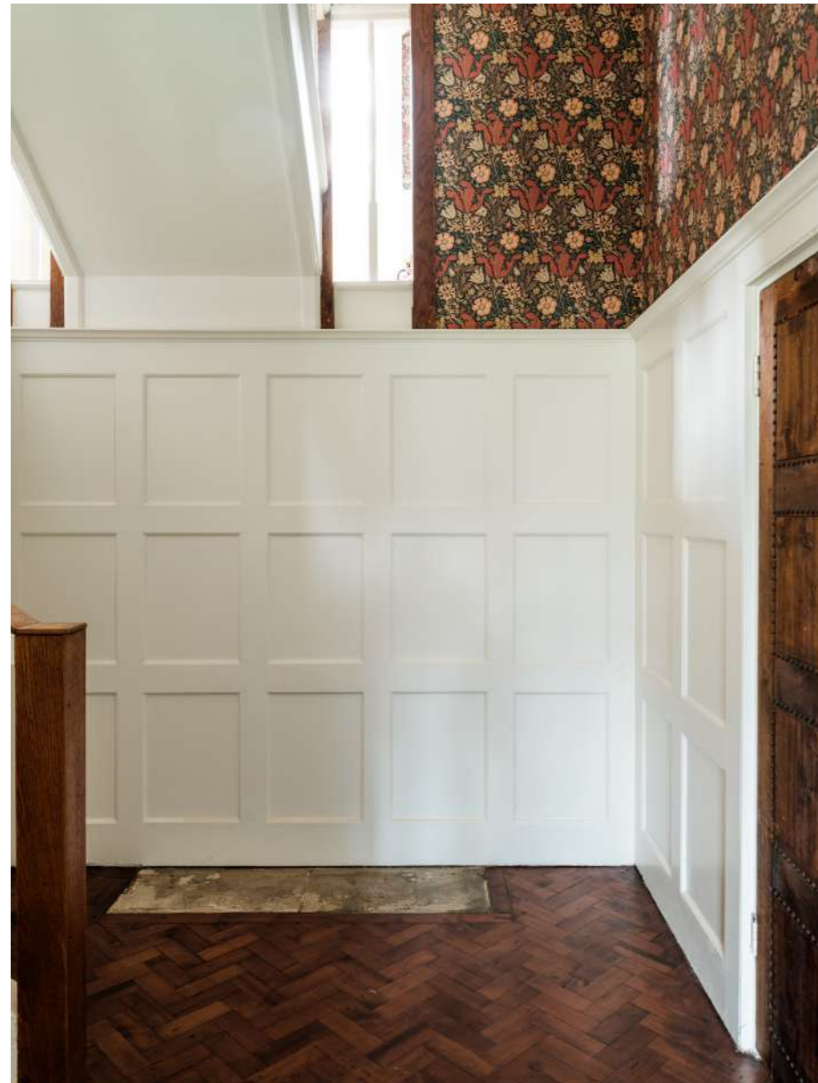
Existing internal panelling to be removed and new sliding screen installed to match the detail of the adjacent sliding screen facing the garden lobby.
