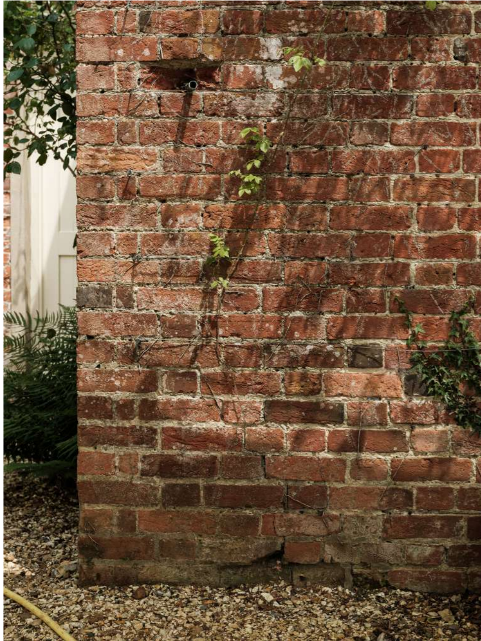
Lean-To Existing structure showing signs of subsidence.
