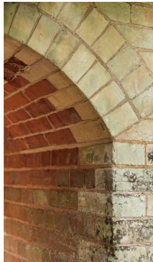
Webb deployed the use of 'Beaulieu buff' bricks to face Nash original house
