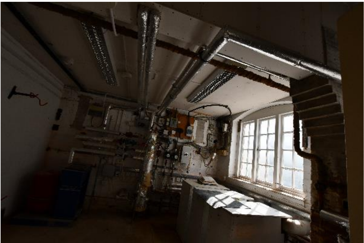
Image 4 Internal view of boiler house
