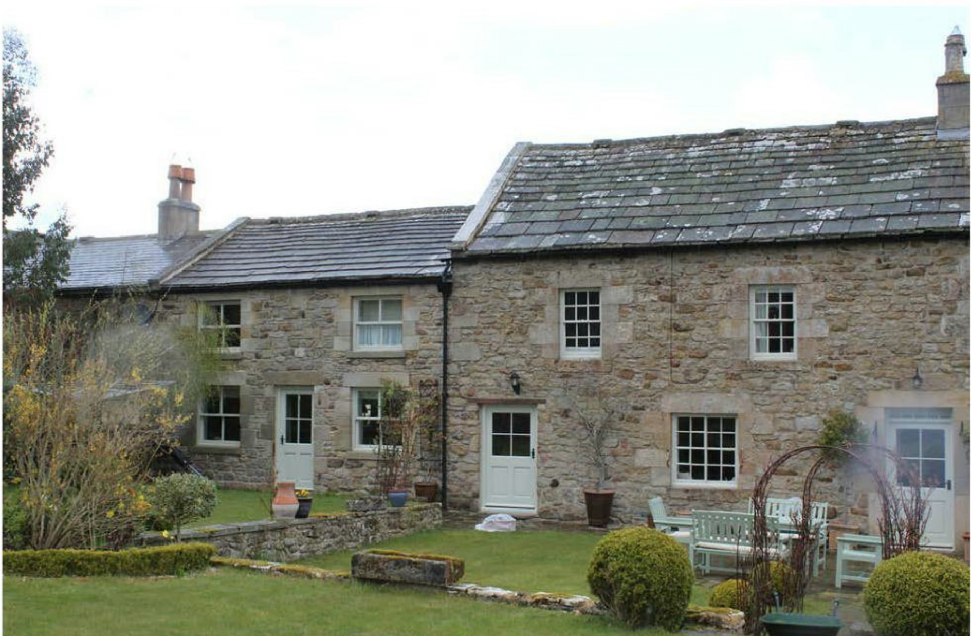
Figure 12 View of western extent of farmhouse range, including inserted doorway in context with other openings
