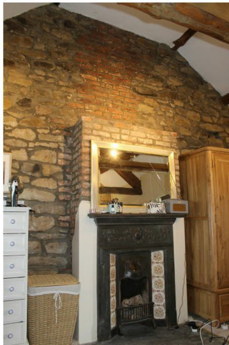
Figure 16 View of faux fireplace against internal, first-floor, east gable wall of farmhouse range
