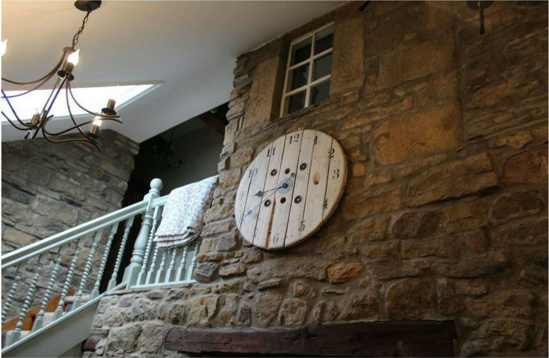
Figure 13 Opening for galleried landing, note evidence of historic structural development to right
