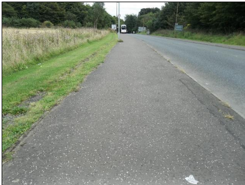
Footway provision along the northern side of the B6392 Gilmerton Road looking eastwards from the A7 Gilmerton Road roundabout
