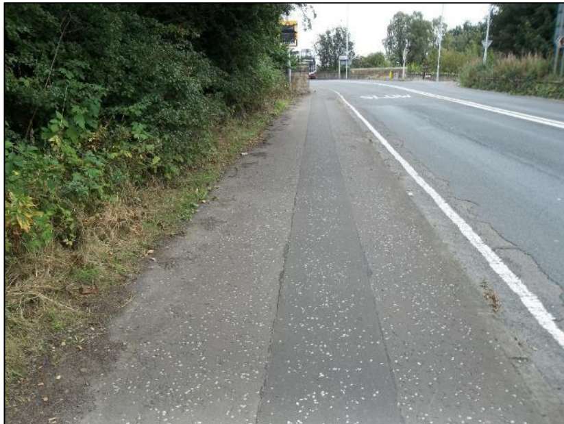
Footway provision along the eastern side of Old Dalkeith Road looking northwards towards Melville Gate Road from the southbound bus stop
