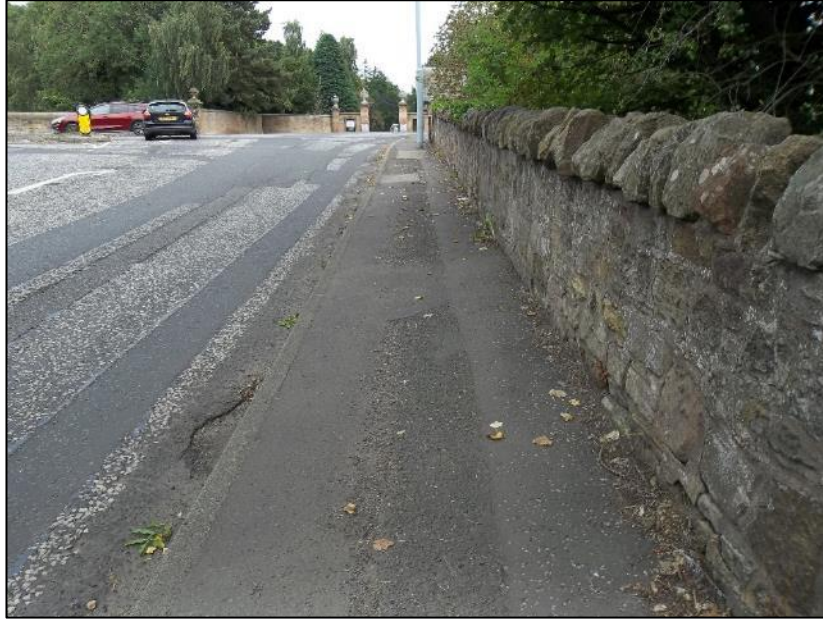
Footway provision along the eastern side of Melville Gate Road looking toward the A6106 Old Dalkeith Road
