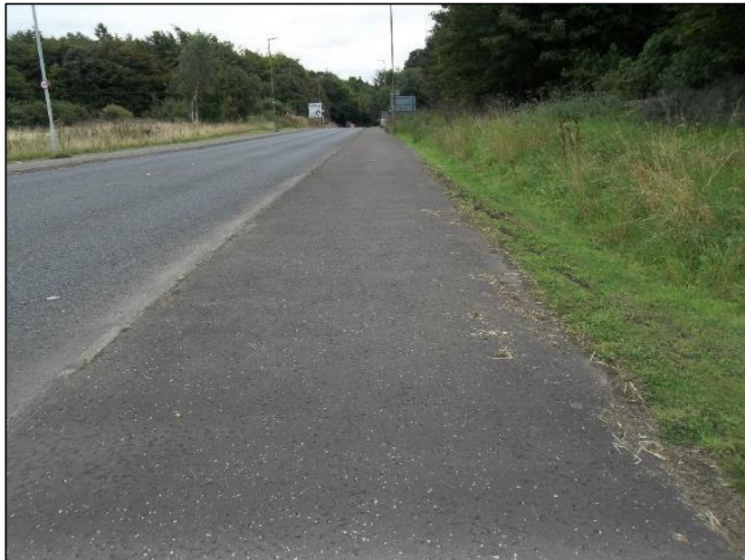
Footway provision along the southern side of the B6392 Gilmerton Road looking eastwards from the A7 Gilmerton Road roundabout
