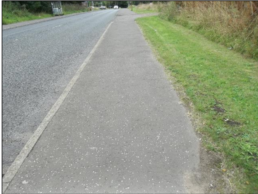
Footway provision along the northern side of the B6392 Gilmerton Road looking westwards with the application site on the right
