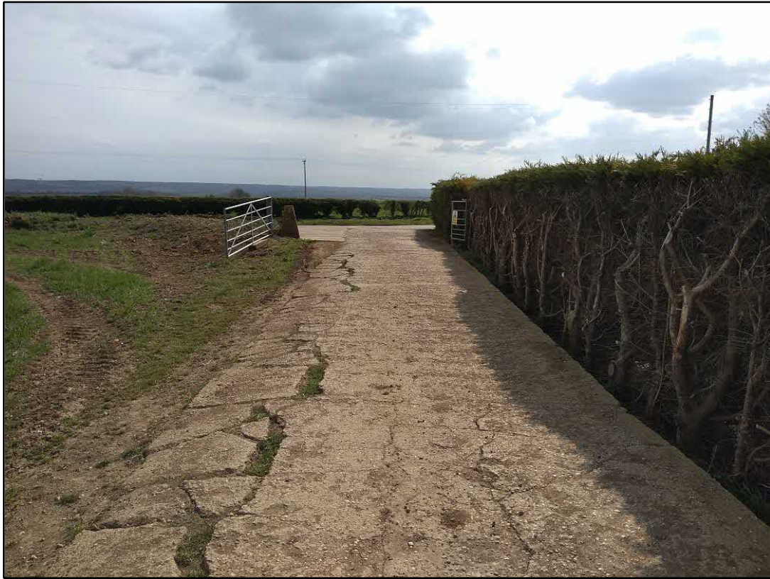
↑ 5) View looking south towards Main Street along existing Farm Access Note severely degraded paving and harsh cutting back of hedgerow
