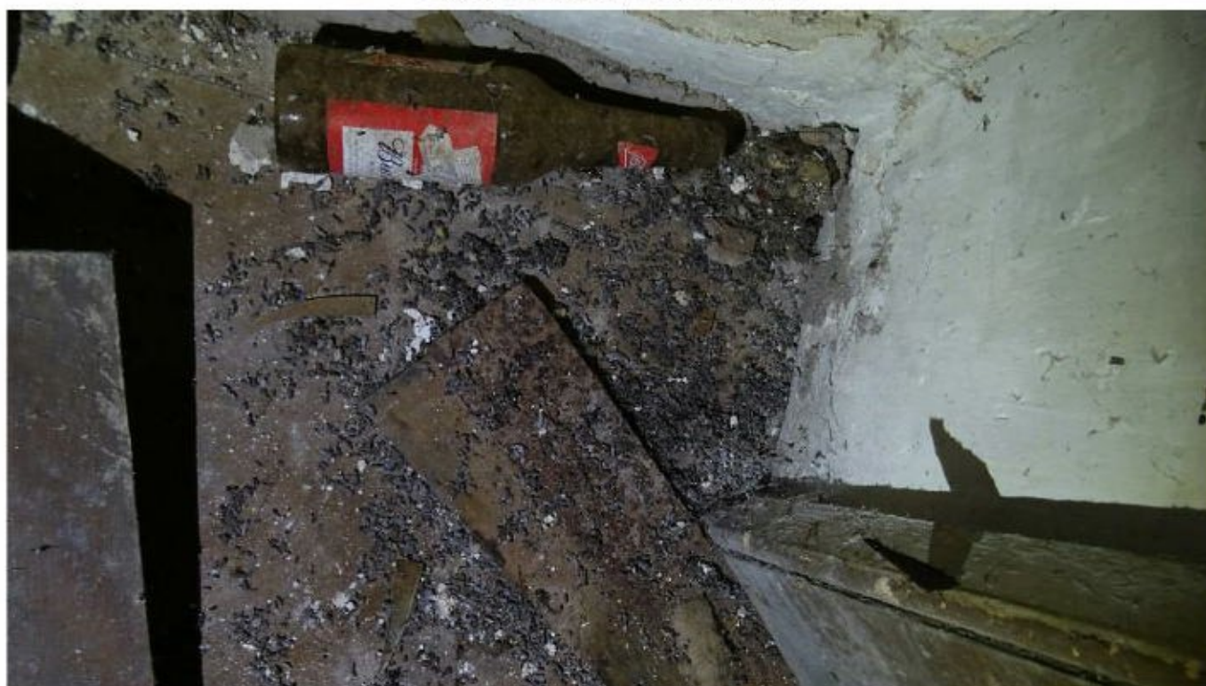
Figure 1.3. Droppings beneath hatch
