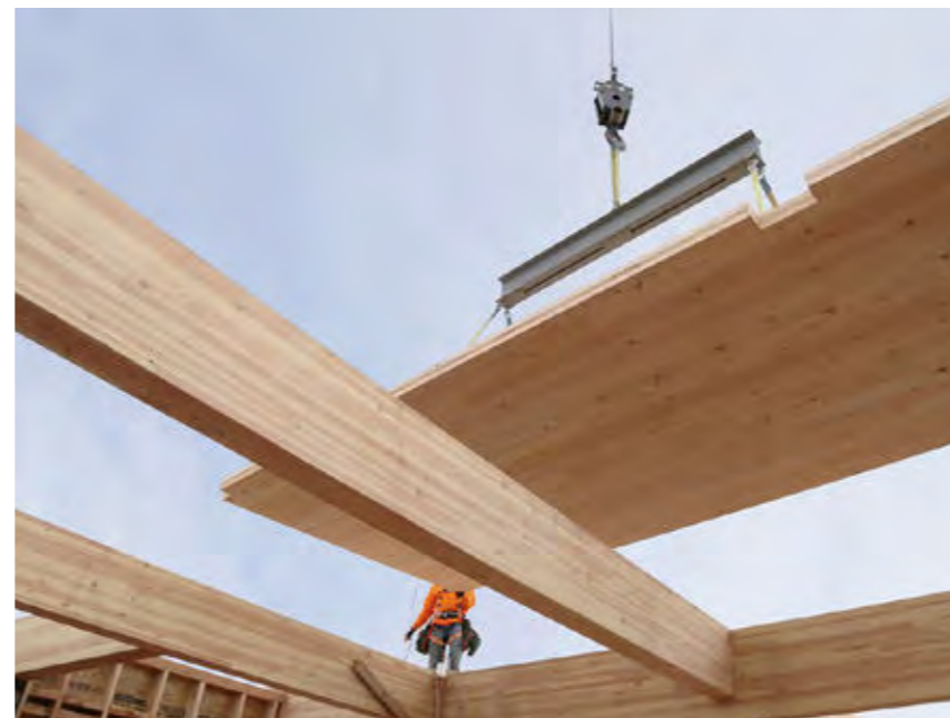
Timber is the primary structural material used across the building for both walls, floors and roof. Whilst thicker than the equivalent support in steel or concrete, the use of timber throughout is a significant reduction in embodied carbon.
