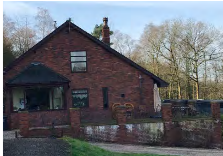
1. The plinth imposes significantly on the landscape and has weathered poorly, detracting from the surroundings.
