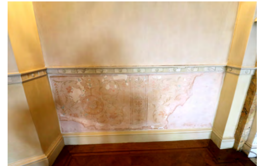
The section of decorated dado adjacent to the Drawing Room fireplace dated to the late 19th/ early 20th century - not being painted over.
