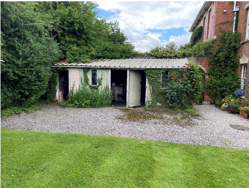
Existing garden stores in a delapidated state
