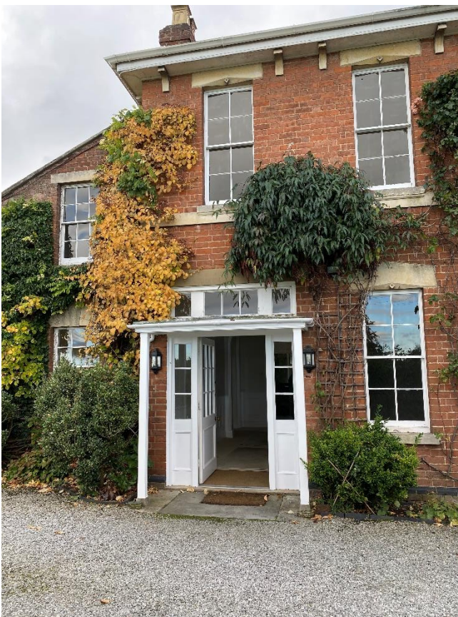
Existing north elevation of the main house with the altered main entrance and insensitive entrance porch – the main entrance would originally have been on the west elevation
