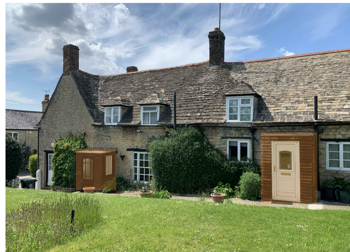
EXISTING MODERN FLAT ROOF TIMBER CLAD PORCHES WITH UPVC DOOR TO BE REPLACED.
