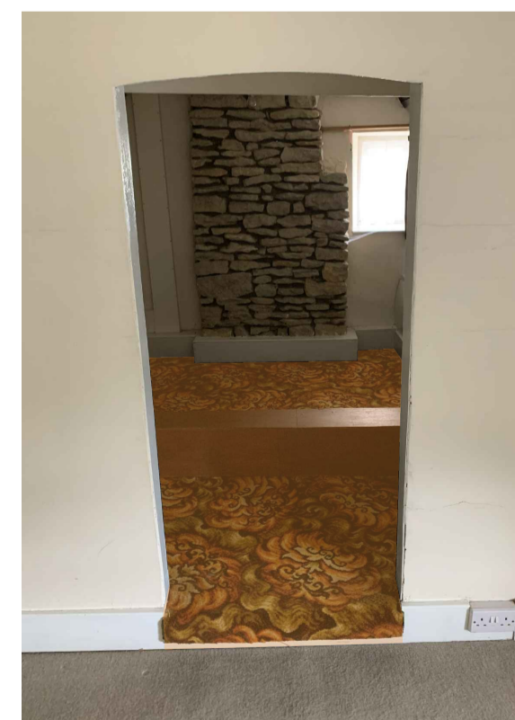
1970'S RAISED FLOOR TO ACCOMMODATE SERVICES AND MODERN RAISED BOXING TO BE REMOVED.
