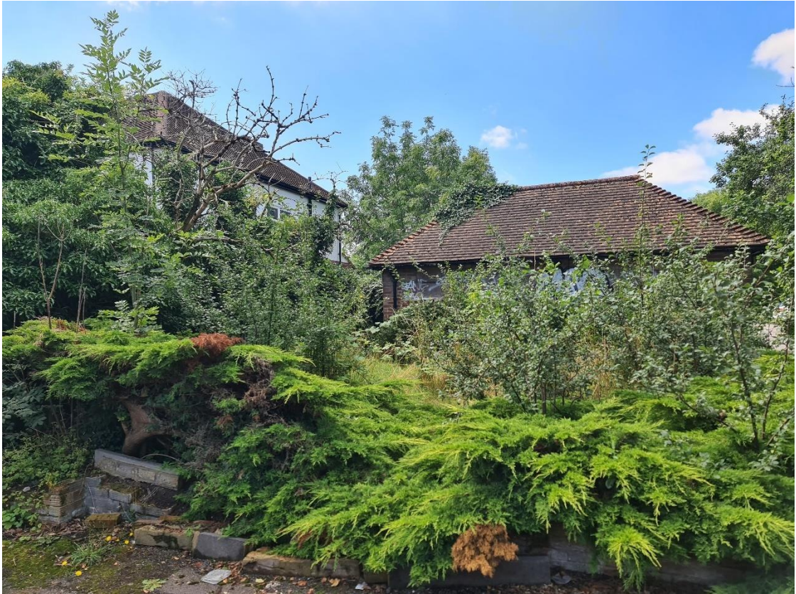
Fig.2: Northeast elevation of the former public toilets and the dilapidated boundary wall.
