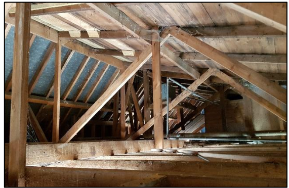
Figure 9: Cluttered roof structure.
