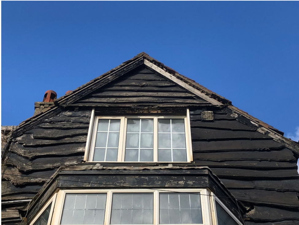
Photograph No.6: Timber cladding to the frontage of No.8 (south Facing), features numerous gaps and lifting where timber has warped.
