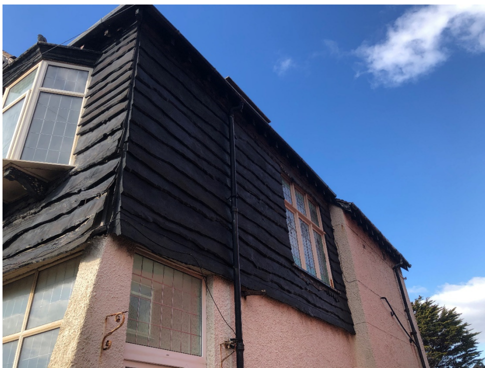
Photograph No.8: Eastern façade of No.8 also has timber cladding present. This is in much better condition than the frontage of the property, but crevices are still present due to the natural unevenness of the timber.
