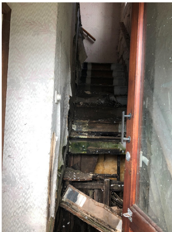
Photograph No.10: showing inside of No.8 Carlin Gate. Stairs have rotted through and much detritus is present on the floors and surfaces.
