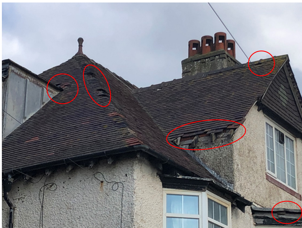
Photograph No.2: Roof of No.6 looking east. Showing damage to roof and lead flashing.
