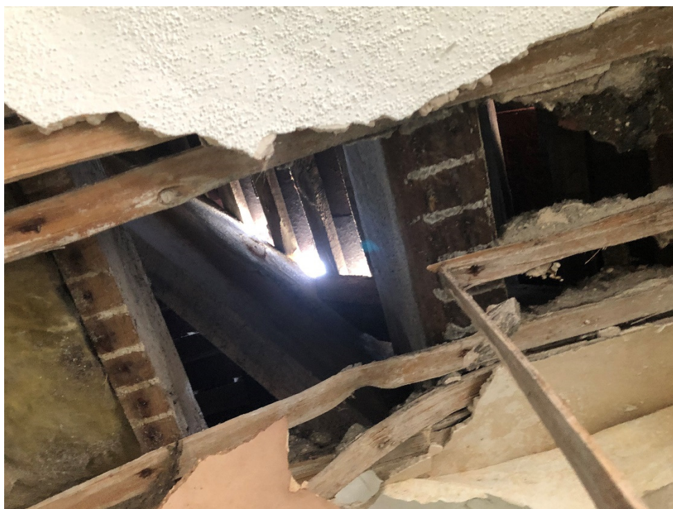
Photograph No.4: Hole in ceiling of attic room, showing tile covering is devoid of underlay and daylight is visible.
