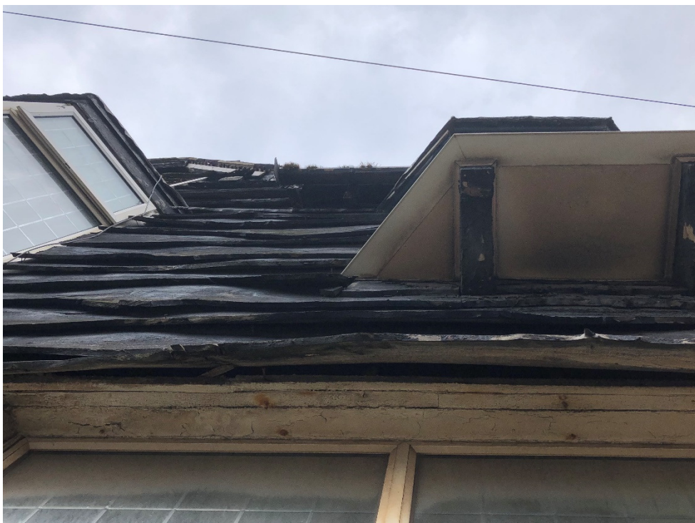
Photograph No.7: showing gaps and crevices under cladding.
