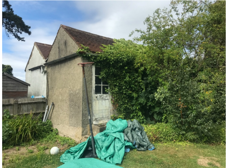
Figure 2: Rear outbuilding in poor condition
