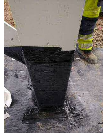
Photograph 18 – An example of some of the detailing around steel columns (Slab E & F)
