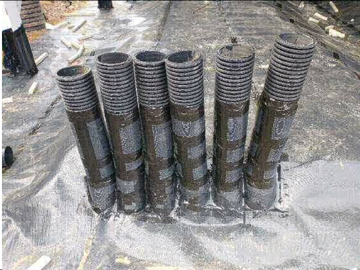
Photograph 17 – An example of some of the detailing around service entries (Slab E & F)
