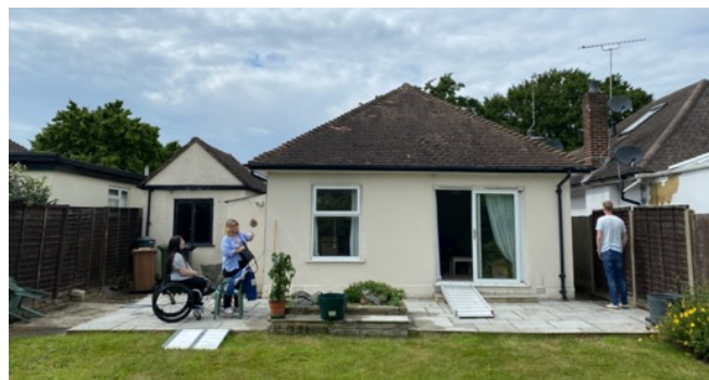
Figure 3: Rear elevation showing roof in poor condition
