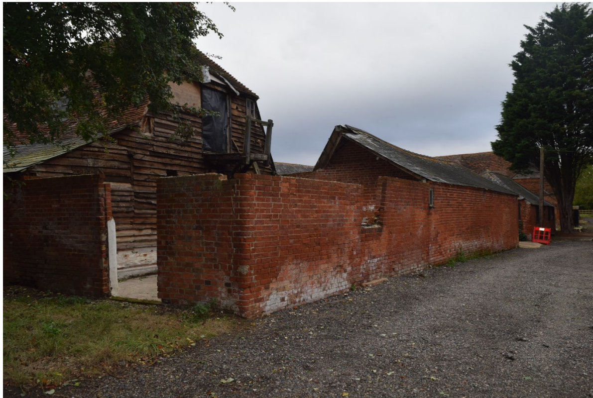
Figure 89: South and East Elevations of the 2-bay open fronted shelter shed and adjacent range.
