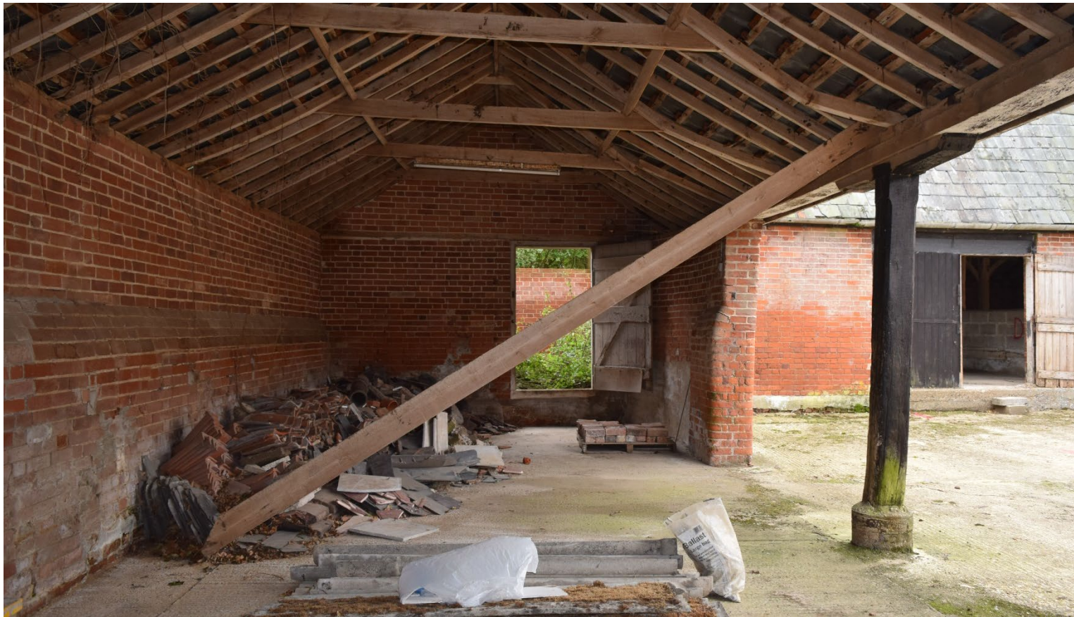
Figure 91: Interior view of the 2-bay open fronted shelter shed. View to the south.
