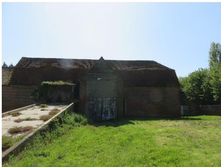
Lean-to adjacent to midstreys porch will be retained and the roof rebuilt to match the existing lean-to on unit 3.
