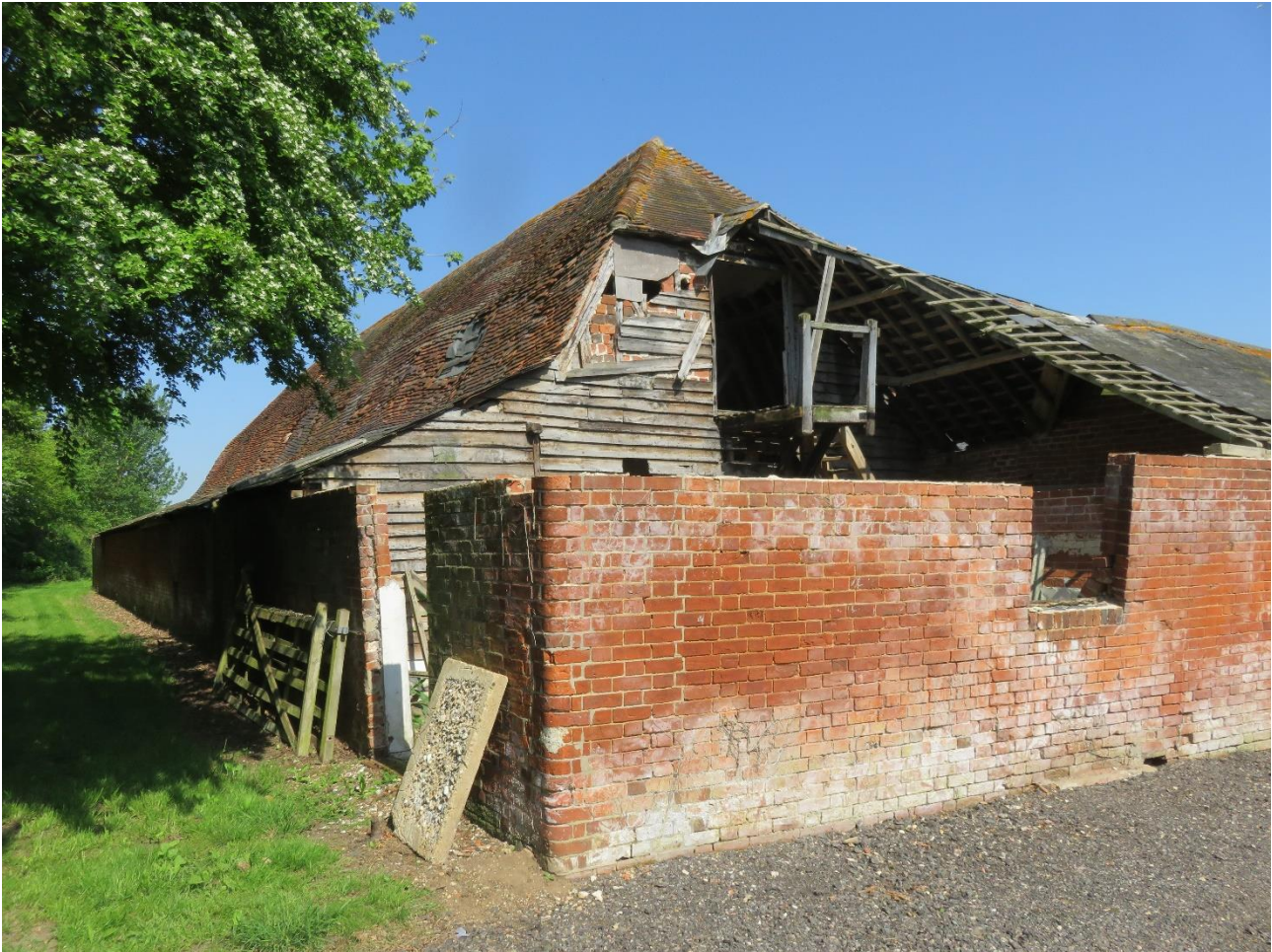
View of east end of Byre, showing collapsed section of roof, which has since been removed.
