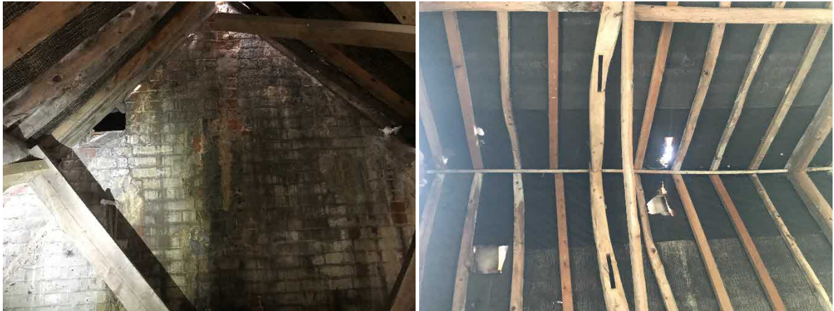
Fig 12 & 13 Gap in east gable wall of dwelling into attic space R2 (left), holes in roof felt and voids in frame (right)
