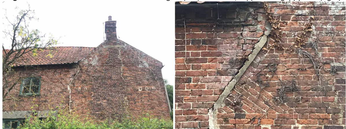
Fig 4 & 5. Vertical brick cracks in west facing elevations of main dwelling (B1)
