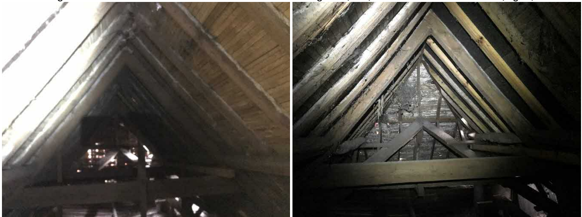
Fig 8 & 9. Internal view of north loft space (left) and gaps at eaves into the loft (right)
