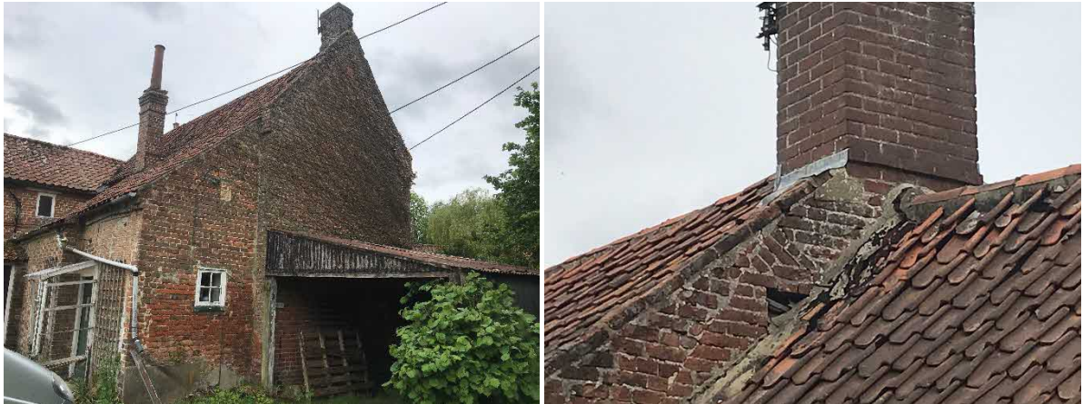
Fig 6 & 7. South and west elevations of building B3 (left) and north elevations (right)
