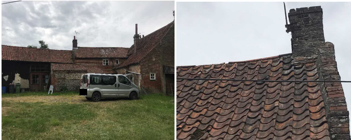
Fig 2 & 3. North and east elevations of dwelling B1 (left) and loose, slipped and gappy tiles (right)
