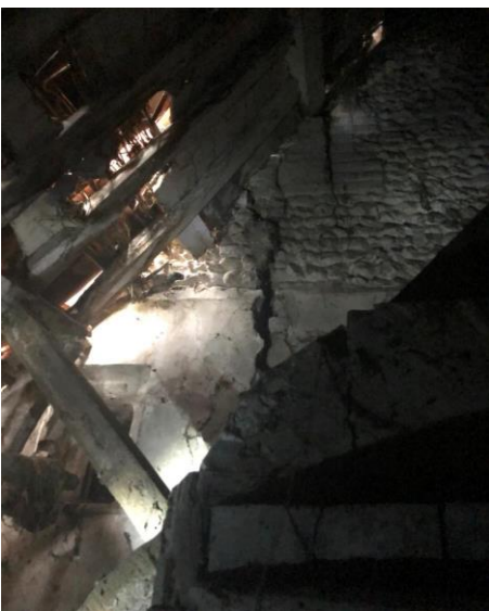
5. Internal first floor - crack to main house east gable
