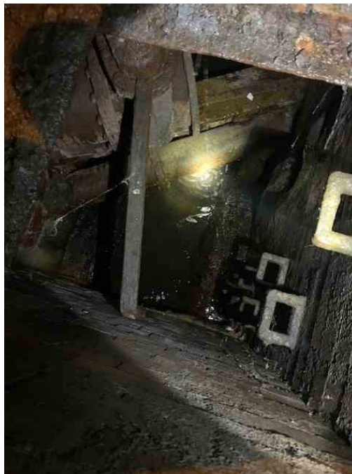
MH03_2c574c19-1a75-486c-8e90-5dc921d056a5_20211214_162501.jpg, 0.00 m General remark
