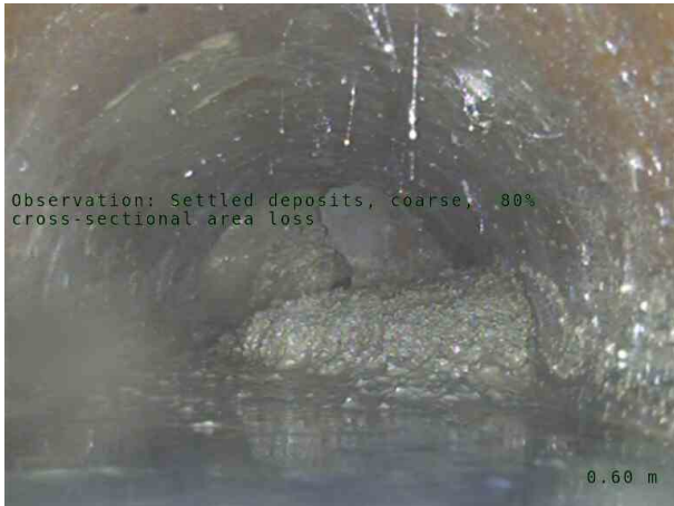
MH01BX_0001.jpg, 00:00:12, 0.60 m Settled deposits, coarse, 80% cross-sectional area loss
