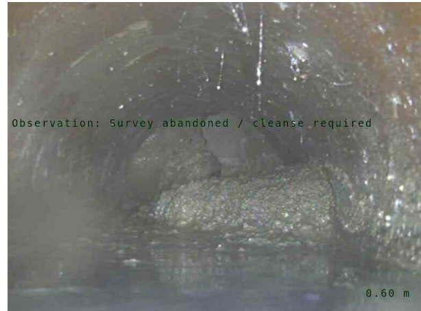
MH01BX_0002.jpg, 00:00:17, 0.60 m Survey abandoned, cleanse required
