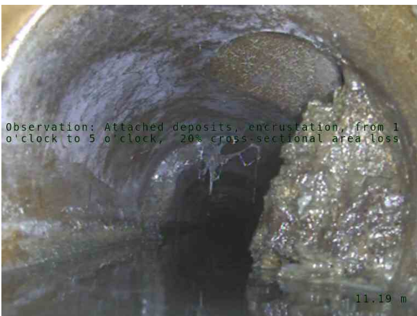
MH01X_0003.jpg, 00:01:45, 11.19 m Attached deposits, encrustation, from 1 o'clock to 5 o'clock, 20% cross-sectional area loss
