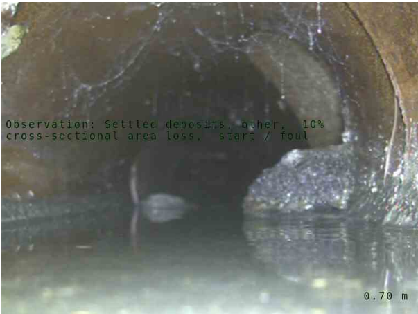
MH01X_0001.jpg, 00:00:13, 0.70 m Settled deposits, other, 10% cross-sectional area loss, start, foul
