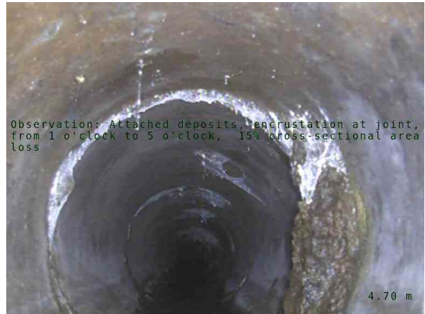
MH01X_0002.jpg, 00:01:09, 4.70 m Attached deposits, encrustation at joint, from 1 o'clock to 5 o'clock, 15% cross-sectional area loss
