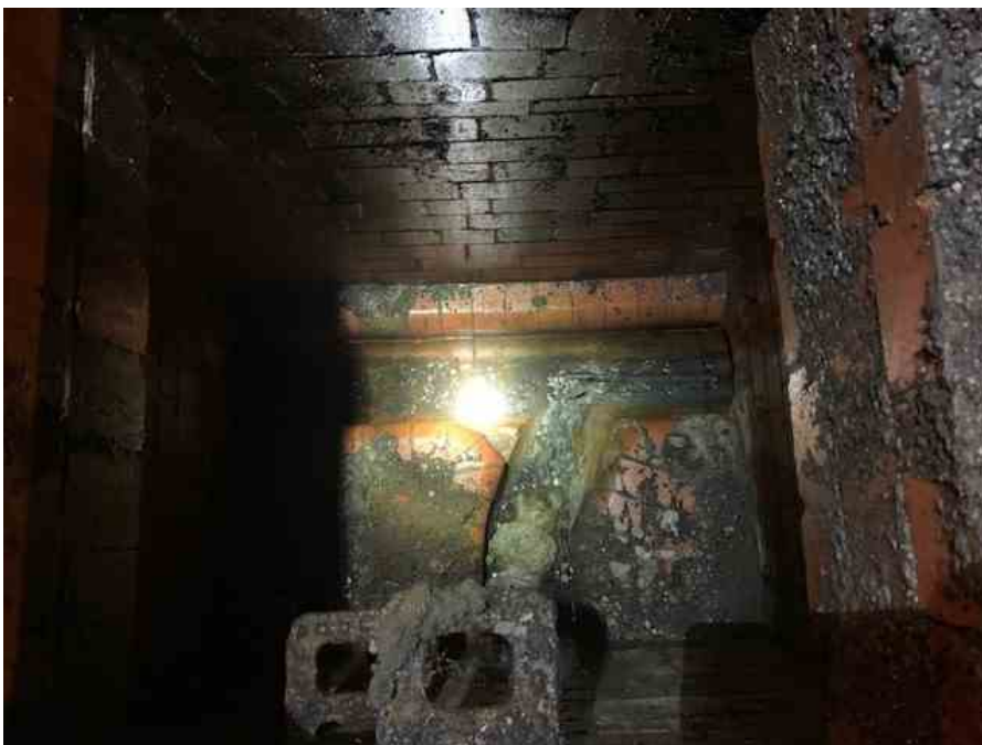
MH02_a1b7d8f5-c5ca-4aa7-9aff-84ebca423ff7_20211214_161613.jpg, 0.00 m General remark
