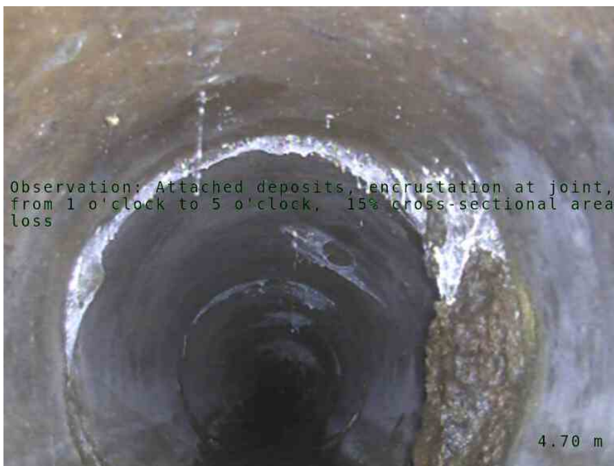
2, 00:01:09, 4.70 m Attached deposits, encrustation at joint, from 1 o'clock to 5 o'clock, 15% cross-sectional area loss
