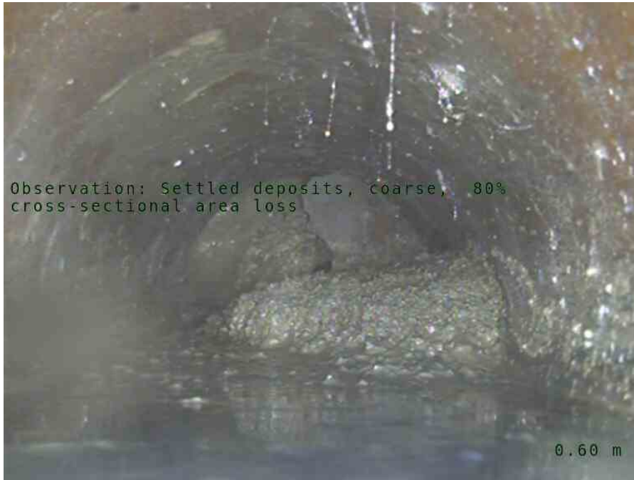
1, 00:00:12, 0.60 m Settled deposits, coarse, 80% cross-sectional area loss
