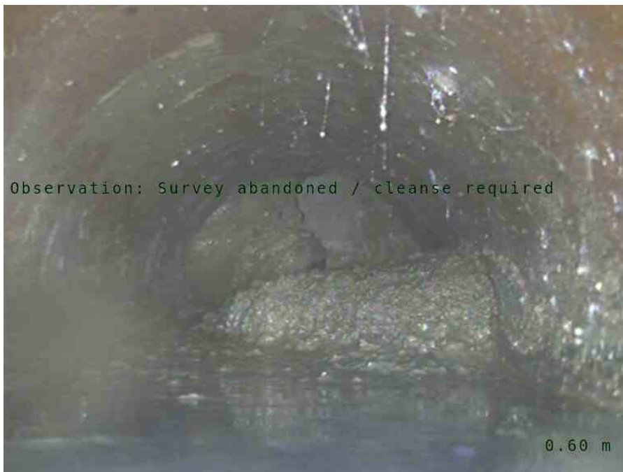
2, 00:00:17, 0.60 m Survey abandoned, cleanse required
