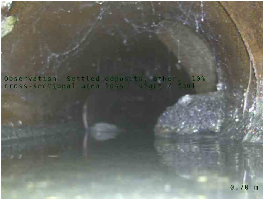
1, 00:00:13, 0.70 m Settled deposits, other, 10% cross-sectional area loss, start, foul
