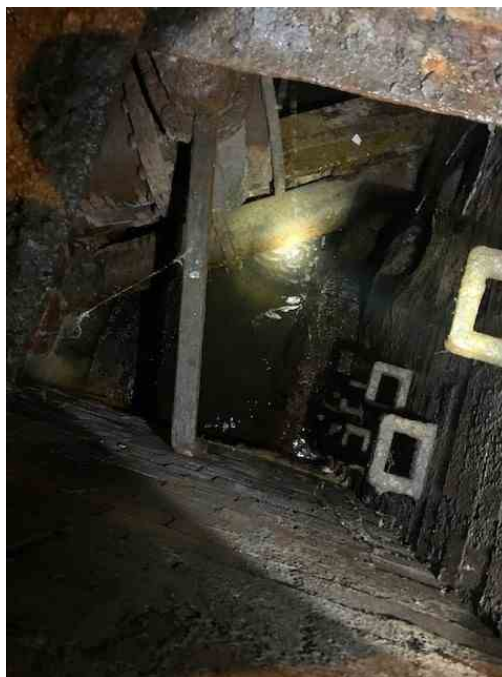
MH03_2c574c19-1a75-486c-8e90-5dc921d056a5_20211214_162501.jpg, 0.00 m General remark
