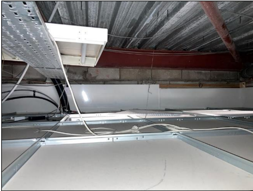
Photograph 17 showing the void space
