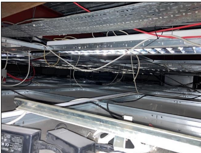
Photograph 18 showing the void space
