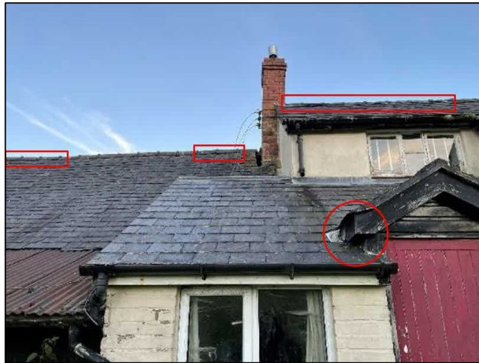
Plate 14. Gaps behind barge board and around chimney on north-eastern elevation of farmhouse
