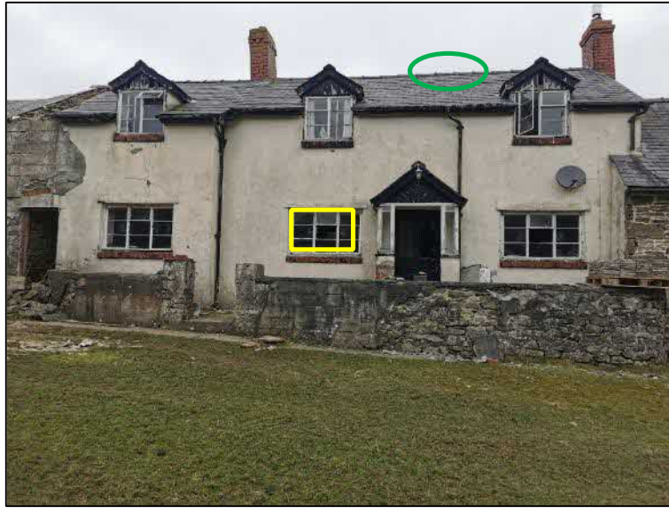
Plate 26. Location of emerging Soprano Pipistrelles via broken window (yellow rectangle) and location of emerging Common Pipistrelle from lifted ridge tile (green circle)
