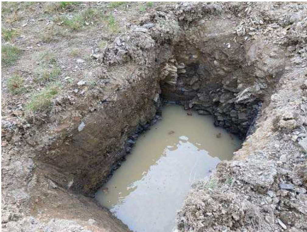
Photograph 18 Description: Trial pit TP02 (end of test) Date: 28/04/2021 Location: North western part of Site A
