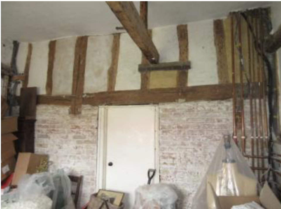
Wall between existing kitchen and back room to be opened up (brickwork removed)
