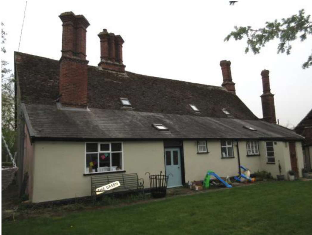
Rear Elevation with existing 20 th Century windows to be replaced – left-hand triple window to be replaced with French doors from Play Room
