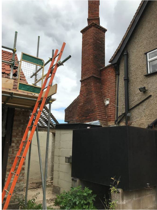
View showing existing blockwork boiler room to be demolished and replaced with a more sympathetic brickwork structure with slate tiling
