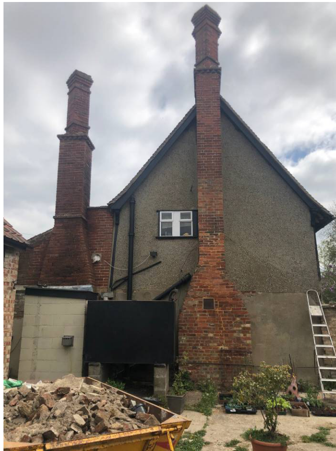
West Gable end – existing window to be replaced & 3 new window openings formed – oil tank repositioned
