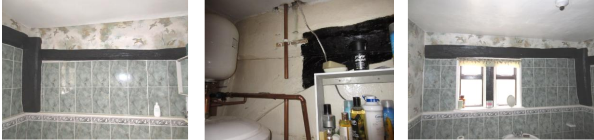
Left: NW corner post with exposed tiebeam (L) and wall plate (R); Centre: arch brace in airing cupboard; Right: 20th century stained timber casements inserted between studs in W gable
