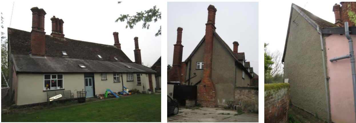
Left: N (rear) elevation showing lean to; Centre: W elevation showing external stacks; Right: E elevation showing junction of main building (pebbledash) with lean to extension (rendered)
