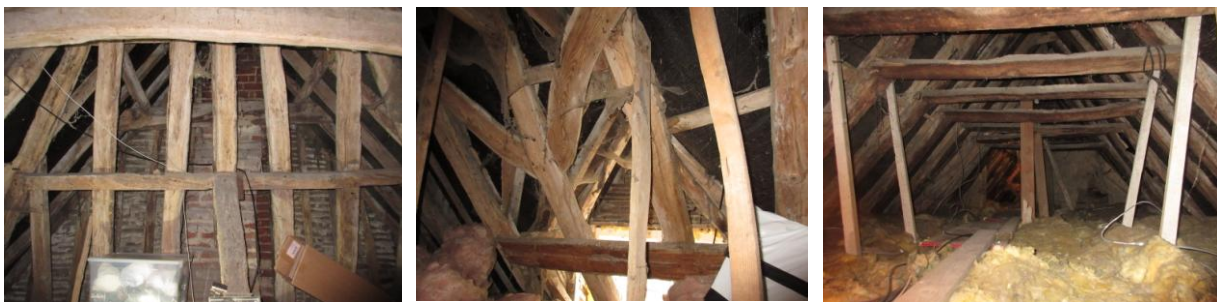
Left: hipped roof structure at W end; Centre: wind braces above dormer; Right: looking E in middle section showing collar rafter roof (no purlins), main stack at end
