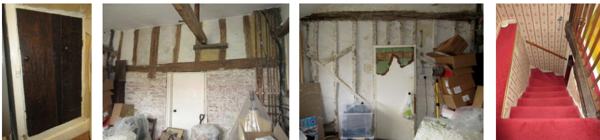
Left to Right: 18th century plank and batten door to understair cupboard in kitchen; N wall (former exterior N wall of main house) of utility room in lean to extension; E wall of utility room with flush door to W hall; W winder staircase with stained wood balusters
