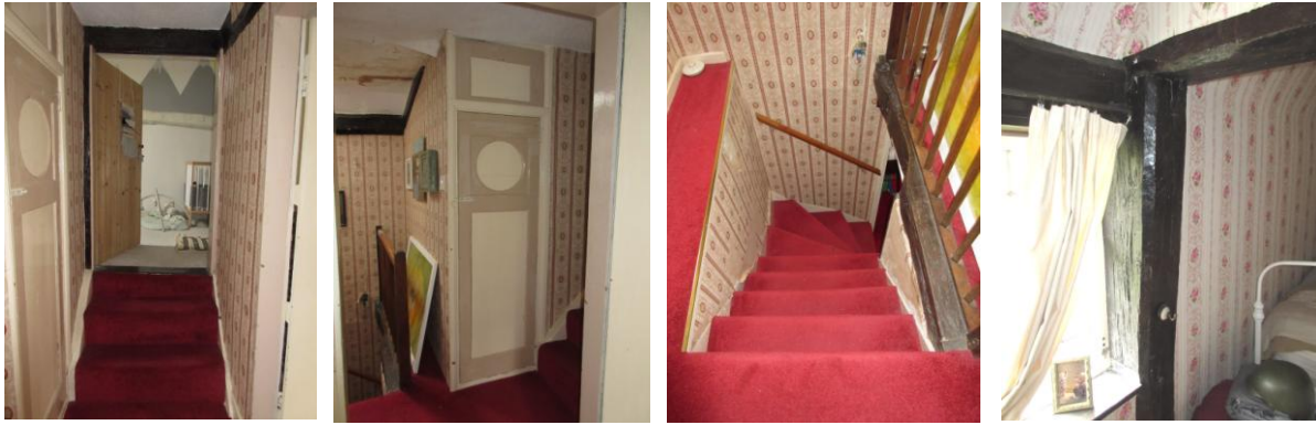
L to R: looking E towards middle bedroom W showing difference in floor level; 1930s panel door to linen cupboard; winder staircase; W bedroom showing exposed mainpost, tiebeam and S wall plate
