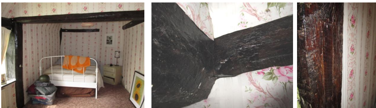
Left: looking W showing exposed tiebeam, S main post and angled NW corner where stack is positioned; Centre: run out stop on axial beam; Right: blocked slot for arch brace in main post
