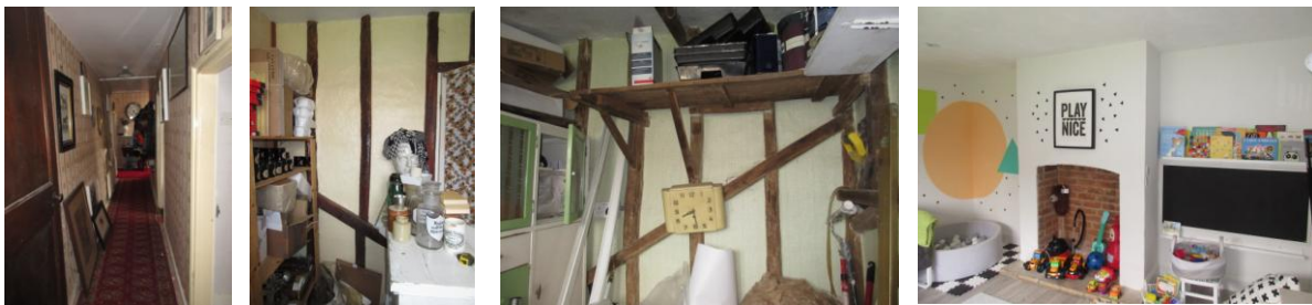
Lean to rear extension, L to R : corridor looking W with studwork wall on right; S wall of former bathroom; S wall of workshop (former larder); S wall of study with disused fireplace
