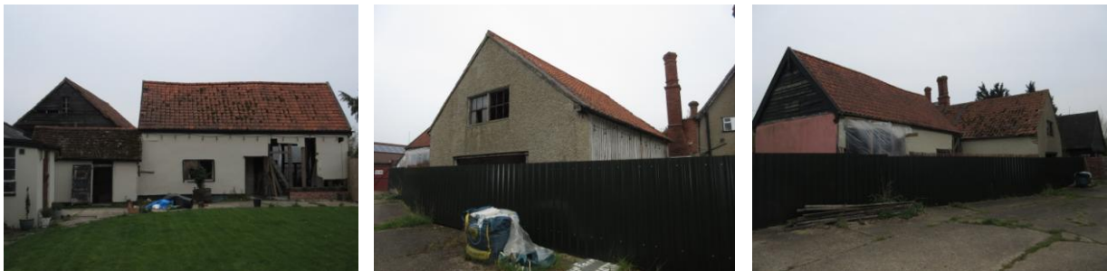
Left: looking W towards coal store (gable of Building B behind), Building A on right; Centre: looking N from access to adjacent property N of Cottage Farmhouse; Right: looking SE from access towards Buildings A & B, Building C visible on extreme right
