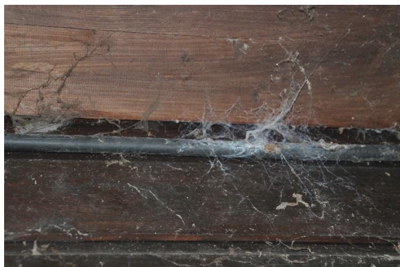
4. Join of soffits and wall covered in cob webs
