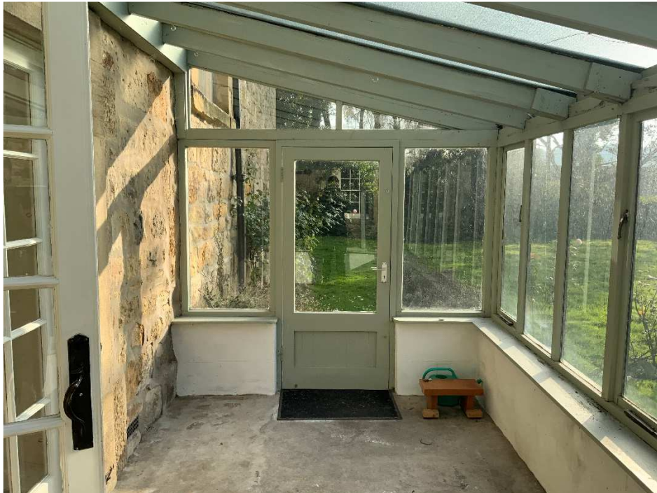
Dilapidated conservatory to be demolished
