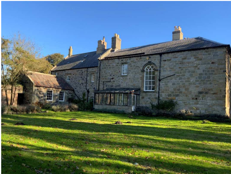
East elevation showing dilapidated conservatory to be demolished
