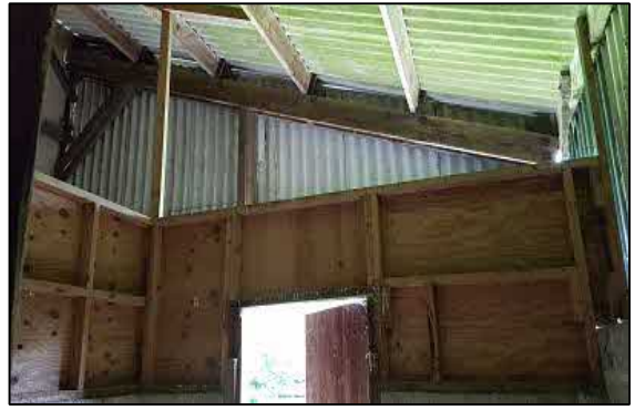
Figure 6: Rear space with wooden partition and unlined roof.
