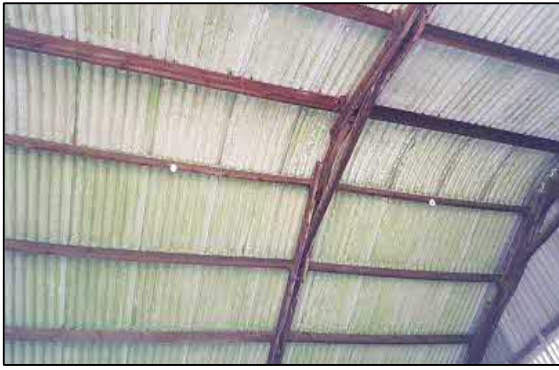
Figure 5: Unlined roof throughout.
