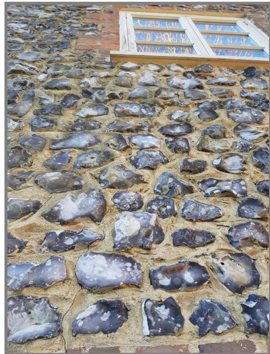
Photograph illustrating the crack extending up to the first-floor window.
