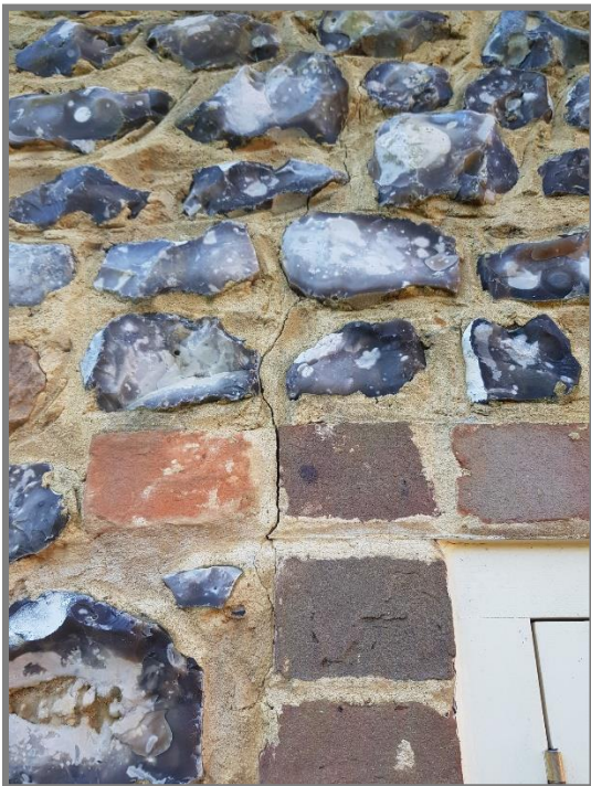
Close up photograph of the crack on the left hand side of a ground floor window
