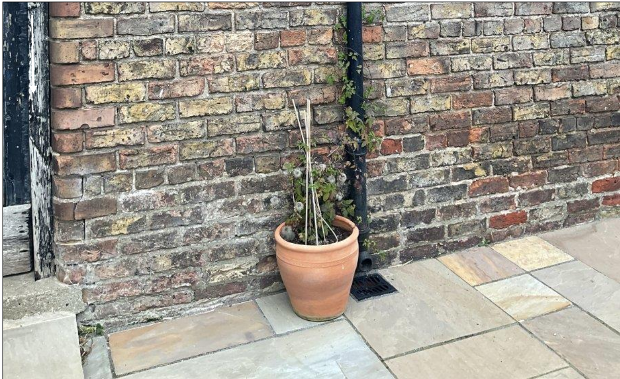
Figure 17 Roof drainage at one of the historic sheds to the immediate east of the farmhouse
