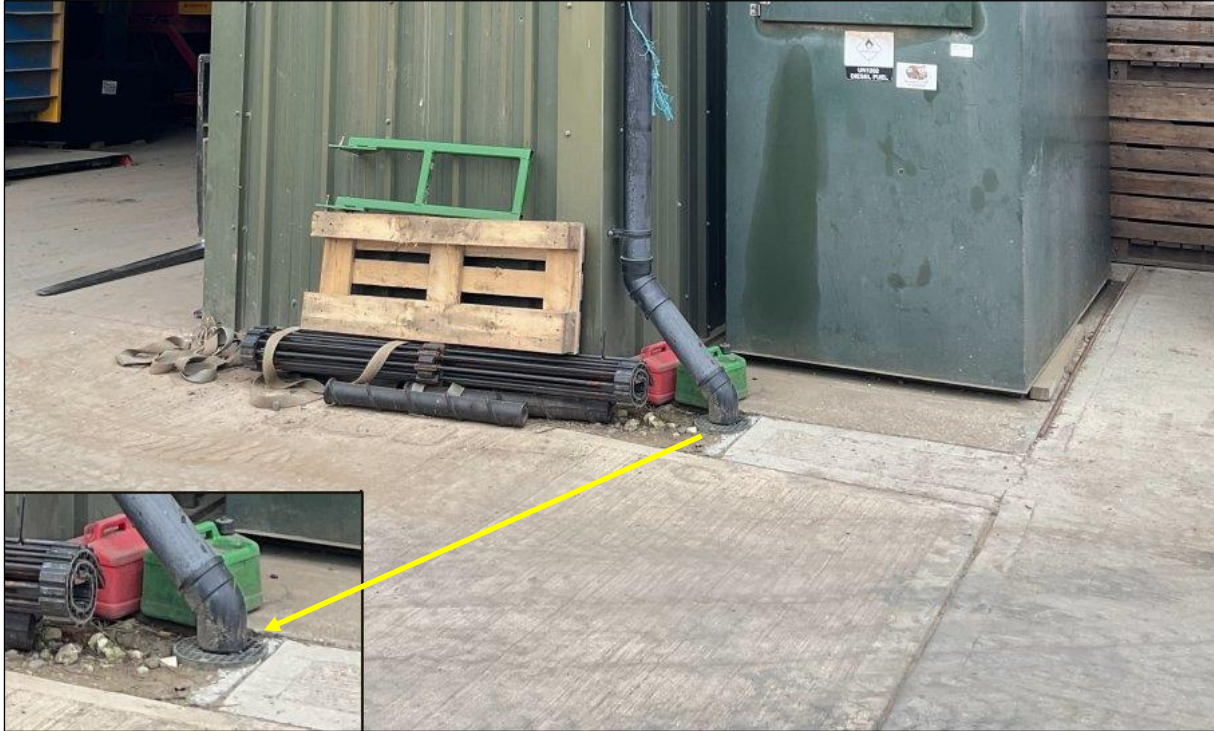
Figure 18 Roof runoff from the new storage building is also plumbed into an underground system
