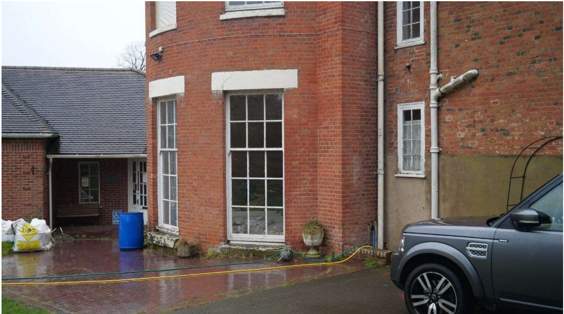
Figure 24: View of South Elevation of Offa House and 1980's Wing and Entrance Doorway
