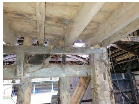
P51 Floor support (Grid C5)
