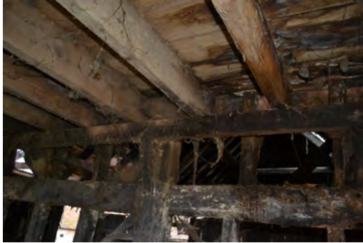
P25 Floor support (Grid C2)
