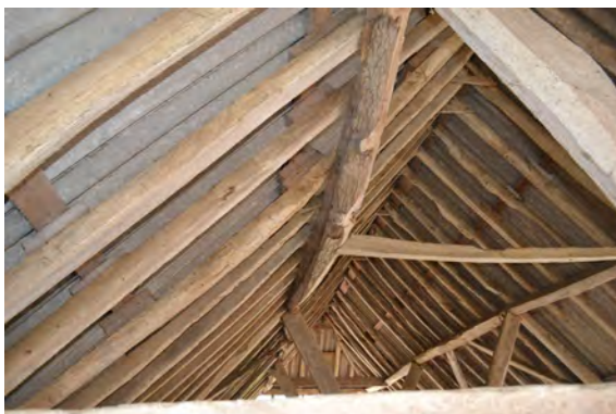
P105 Packing, deflection of purlin
