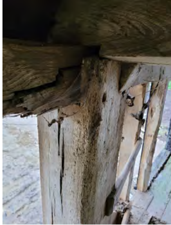
P69 Post split and eaves crack (Grid A7)
