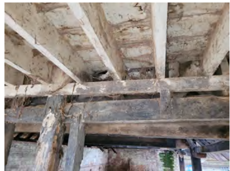
P84 Floor support (Grid C8)
