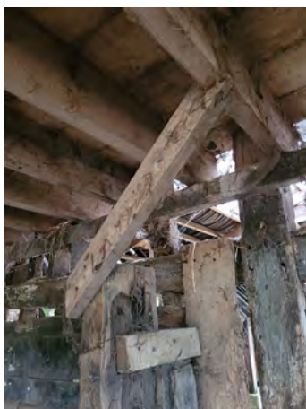
P62 Floor support (Grid C6)
