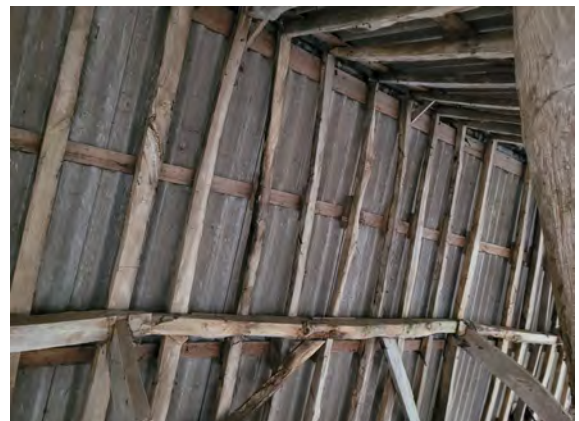
P106 Purlin, brace decay
