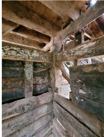
P75 Floor support (Grid C7)
