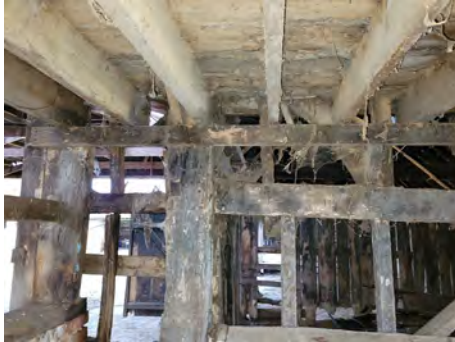
P35 Floor support (Grid C3)
