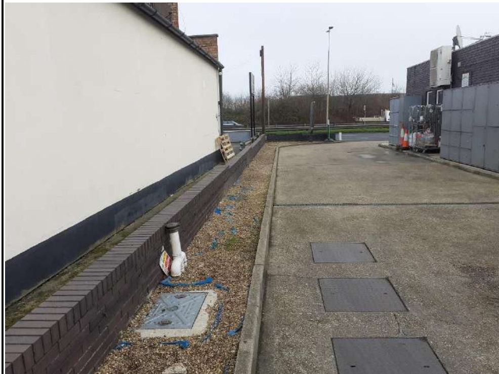
Photo 4: View of defunct carwash interceptor in the southwest of the site.
