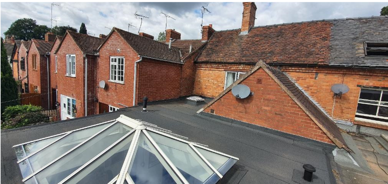
Context Photograph 7: The existing lantern rooflight and felt flat roof to the existing extension c.2015.
