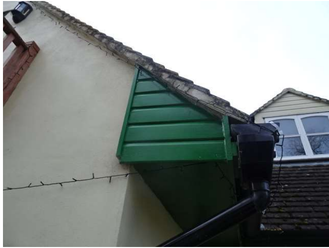
Upper section of front elevation that will be part of the development showing boxed soffits with no gaps to the base or sides.
