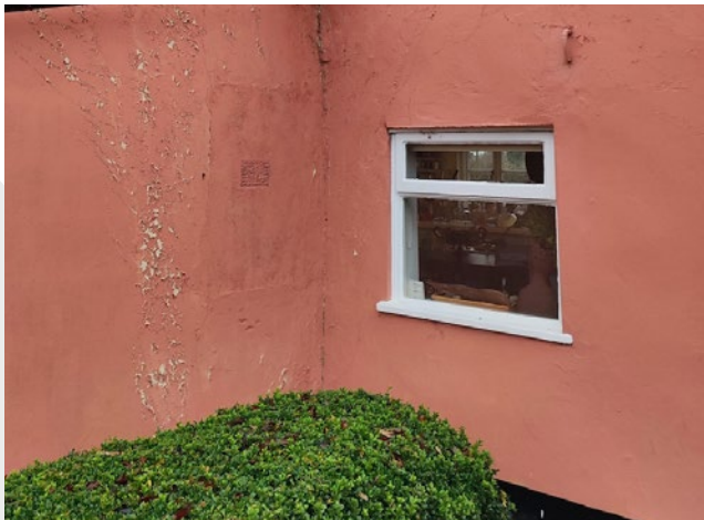
Later addition window to be removed and opening increased to allow for door access to proposed Larder.
