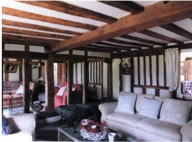
Window to be reinstated in blocked 6-light diamond-mullioned window to dining room.
