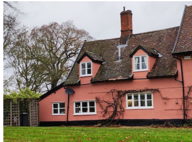
First floor dormer windows to be replaced with timber flush casement slimlite glazed windows. Roof repairs proposed to deal with leaks on this section of roof.
