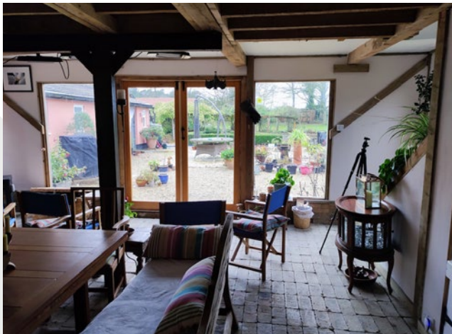
Timber doors to Garden Room to be replaced.
