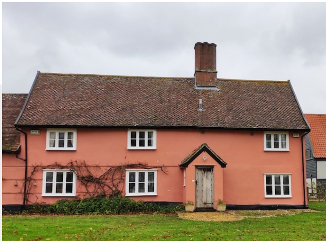
Timber front door to be replaced.
