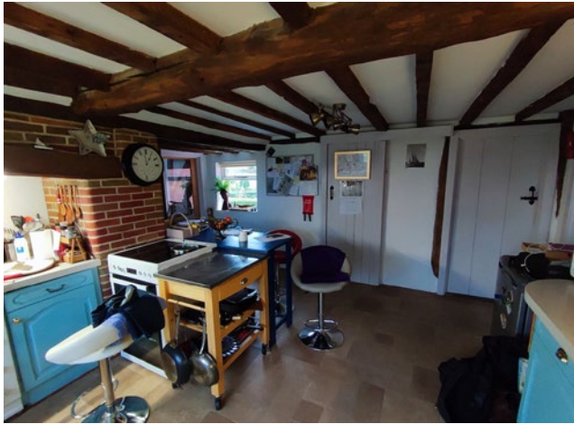
Alterations made to north wall, including removal of modern window and replaced with door opening, existing historic studs to be exposed and doors removed.
