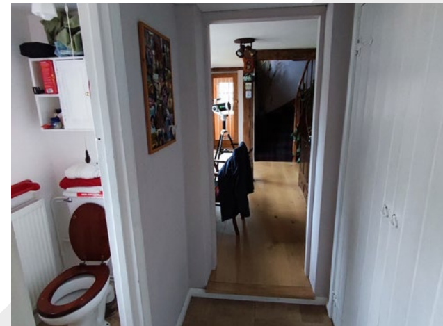
Existing modern cupboards and partition walls to be removed. WC to be altered.
