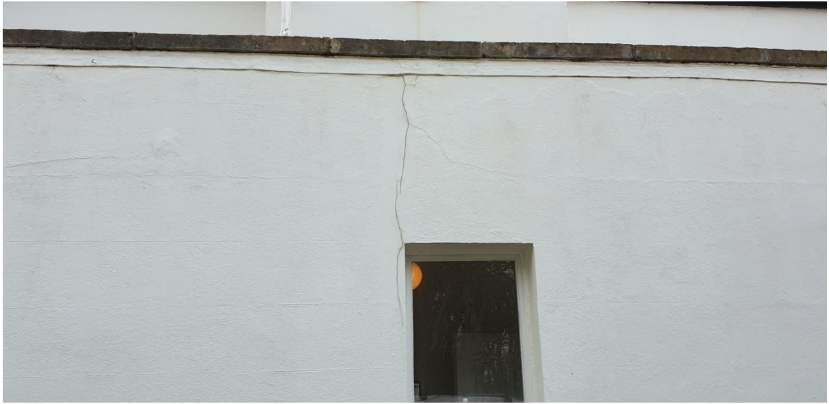
Figure 8: north west damage
