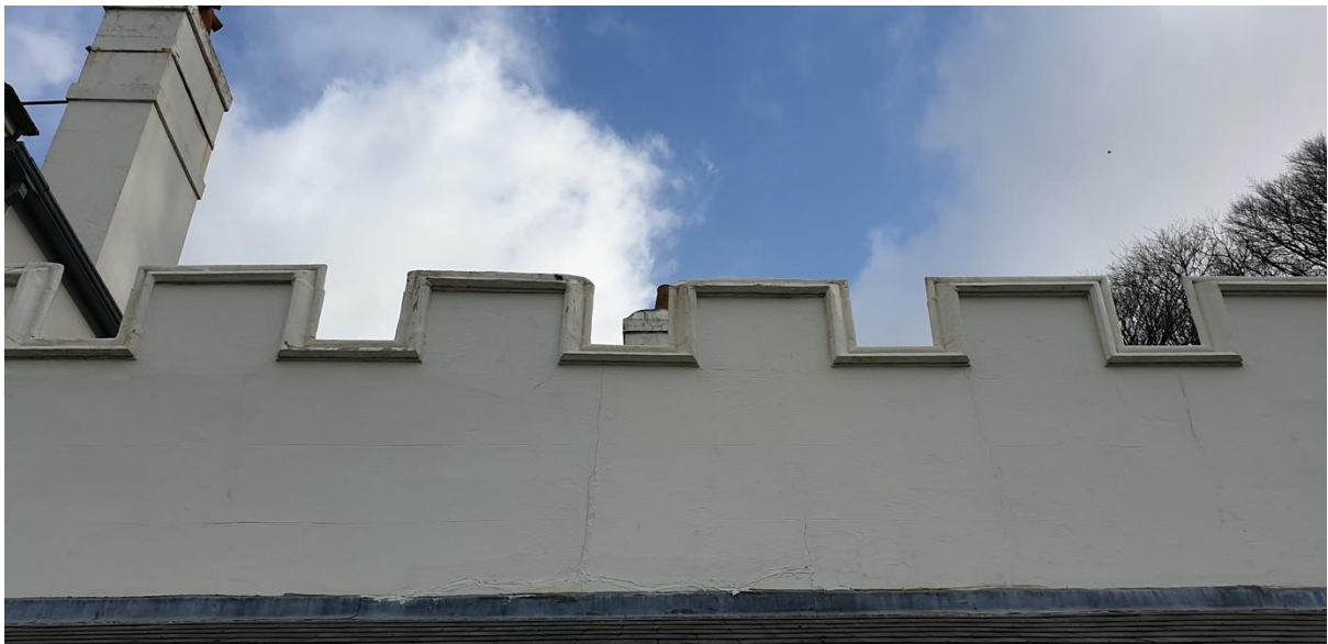
Figure 5: south west damage
