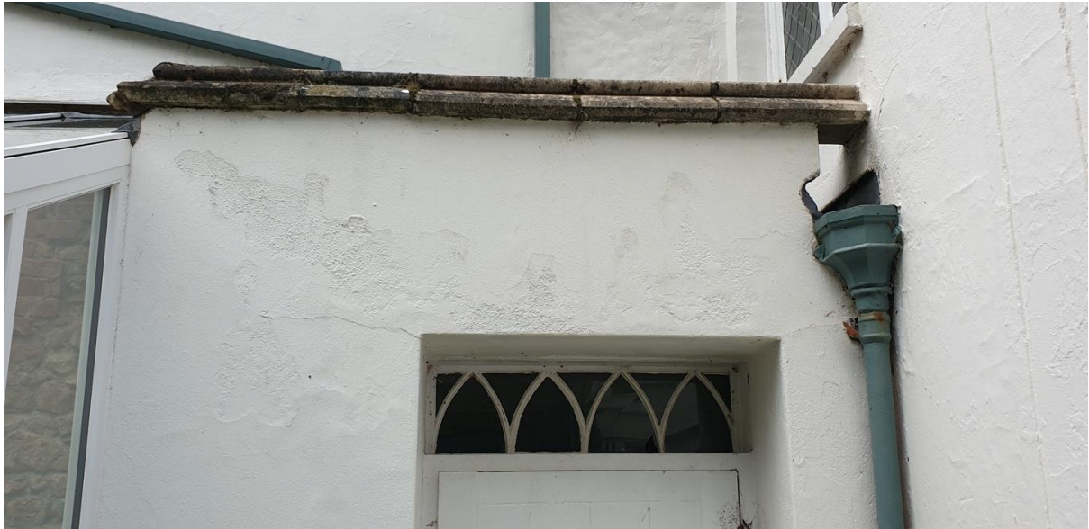
Figure 11: north east damage
