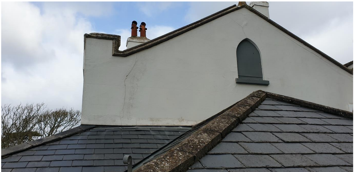
Figure 7: south east damage
