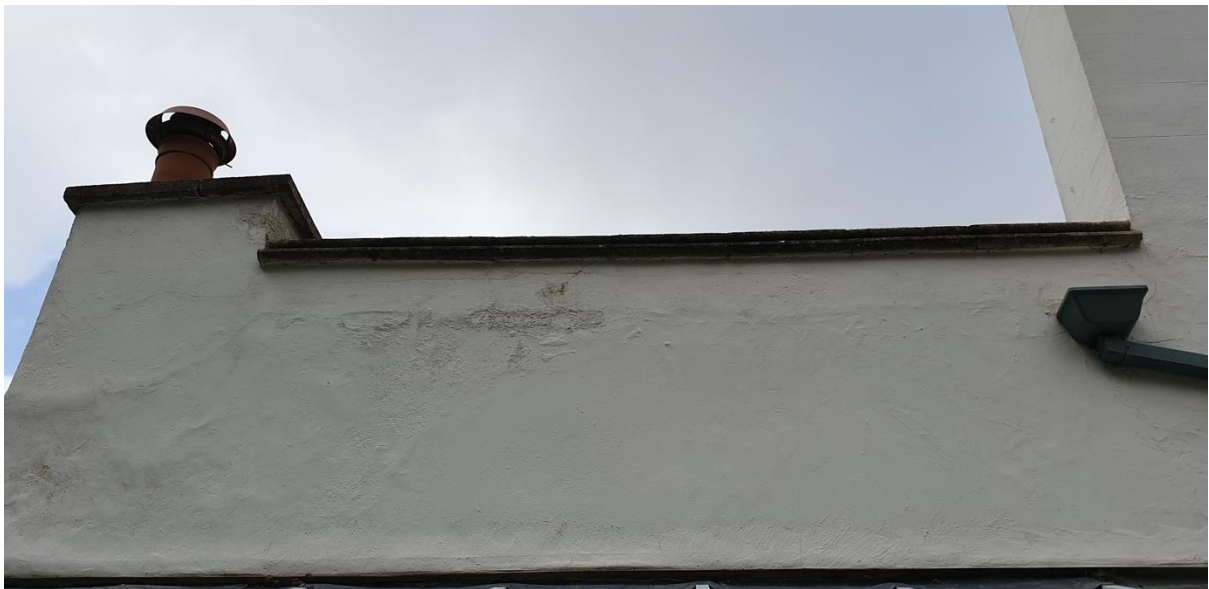
Figure 12: north east damage
