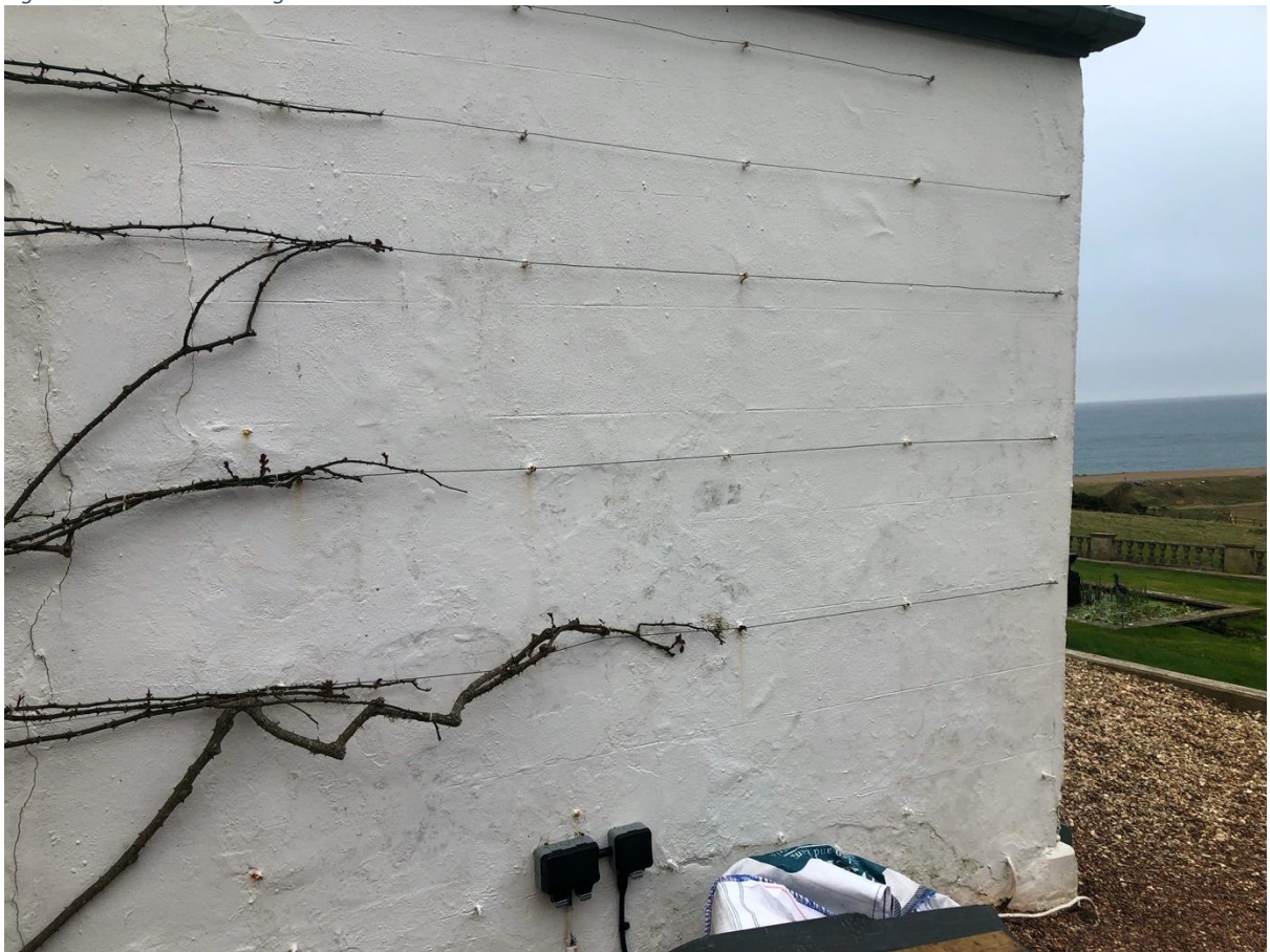
Figure 9: north west damage
