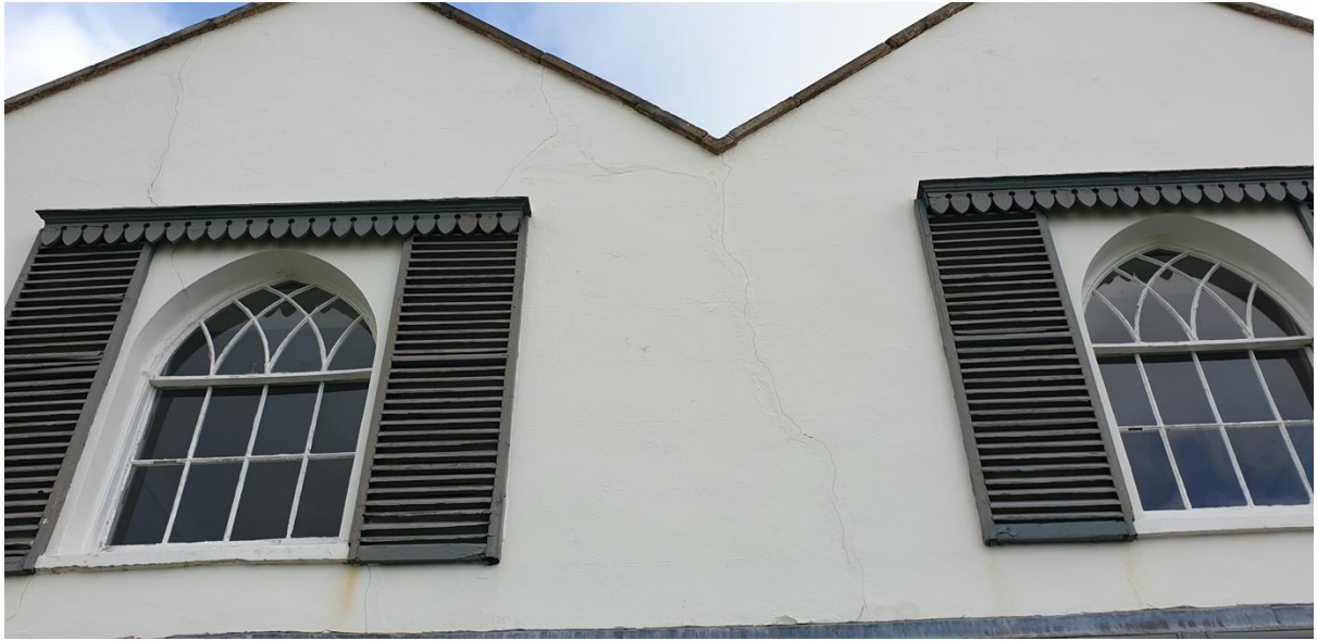
Figure 6: south west damage
