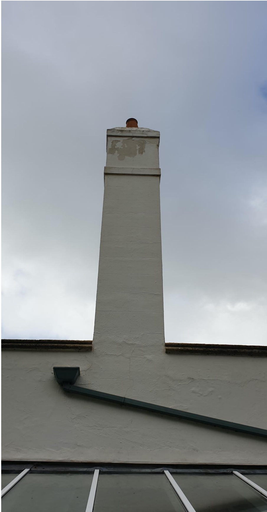
Figure 10: north east damage
