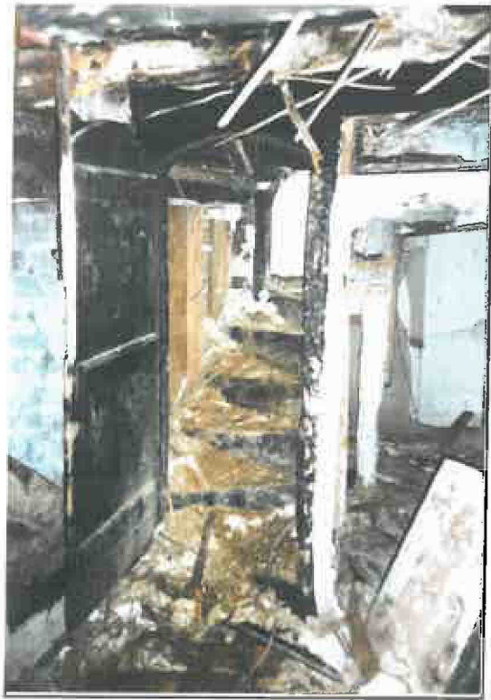
Central Staircase : A considerable accumulation of moisture trapping detritus lay on each tread
