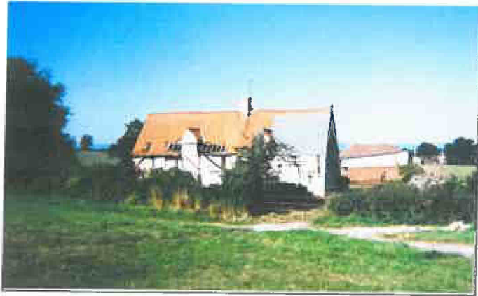
Yew Tree Farmhouse From Whaddon Green, showing large areas of damaged roofing allowing catastrophic water ingress
