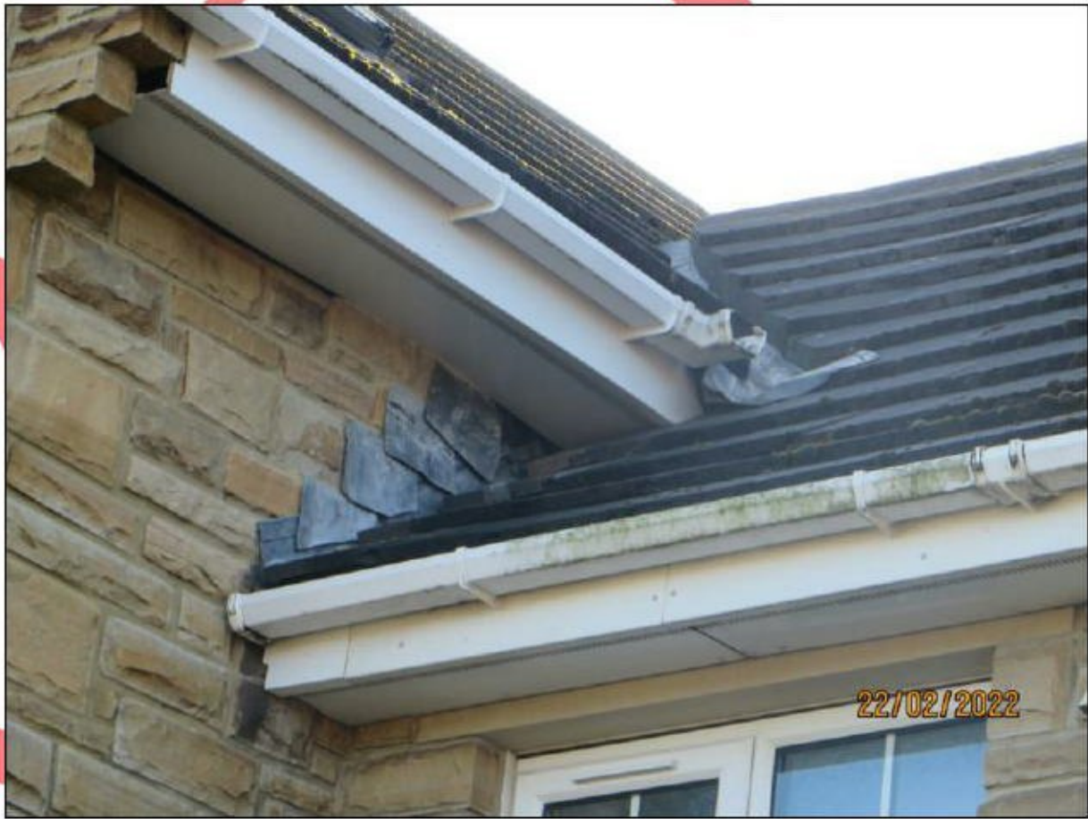
Figure 18. Gap present near soffit box and raised flashing. Not affected by development proposals.
