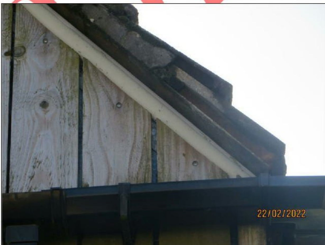
Figure 25. Gap at end tiles on outbuilding.
