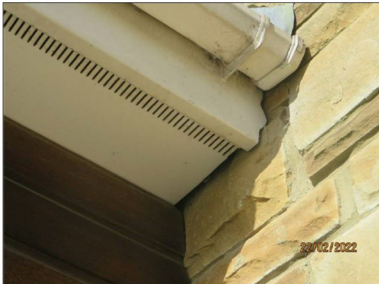
Figure 14. Gap present at end of soffit box on conservatory.
