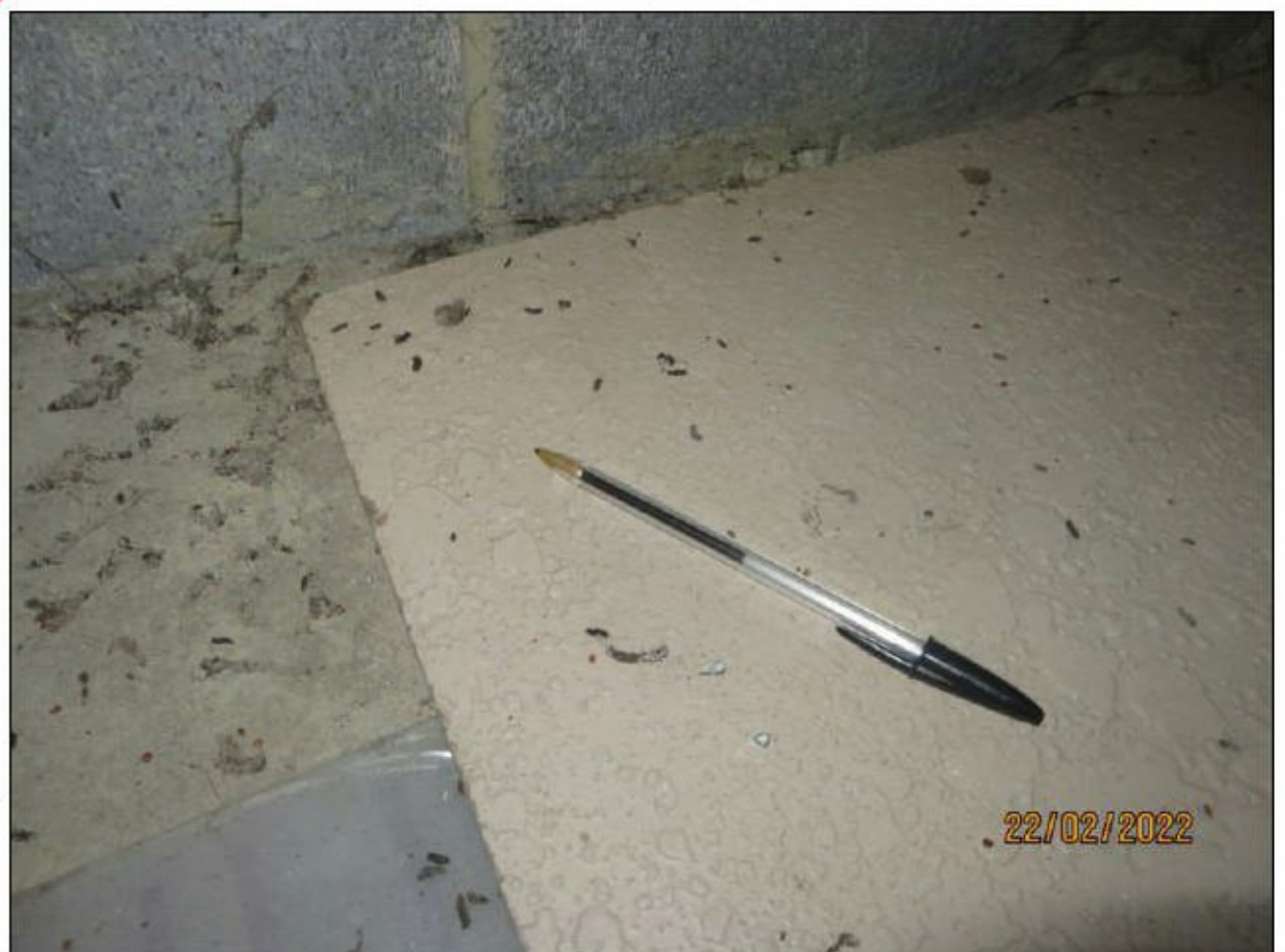
Figure 34. Bat droppings found on upper floor of storage section of outbuilding.
