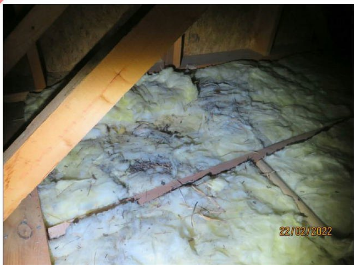
Figure 22. Remains of bird's nest within main house loft void.
