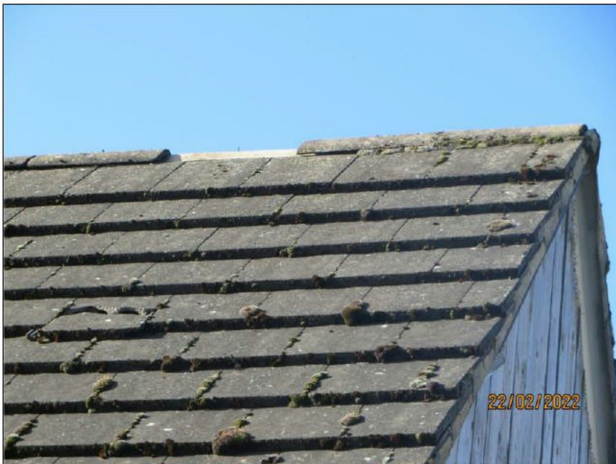
Figure 26. Missing ridge tile on outbuilding.
