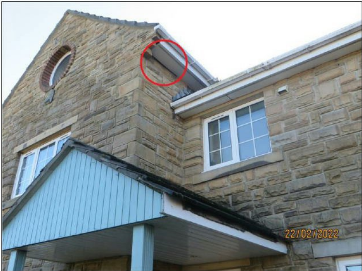
Figure 17. Gap present near soffit box. Not affected by development proposals.
