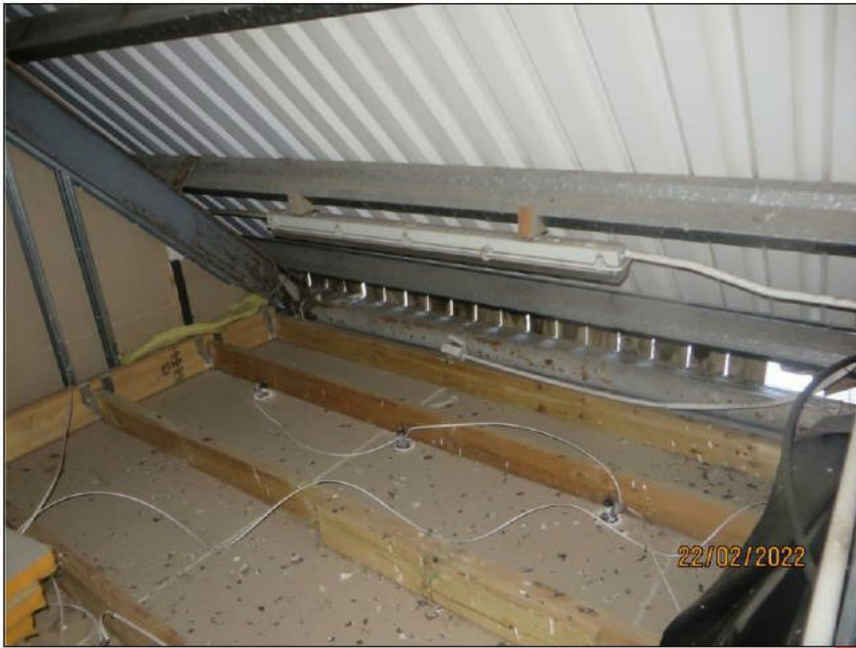
Figure 35. Bird droppings above 'Granny annex'.
