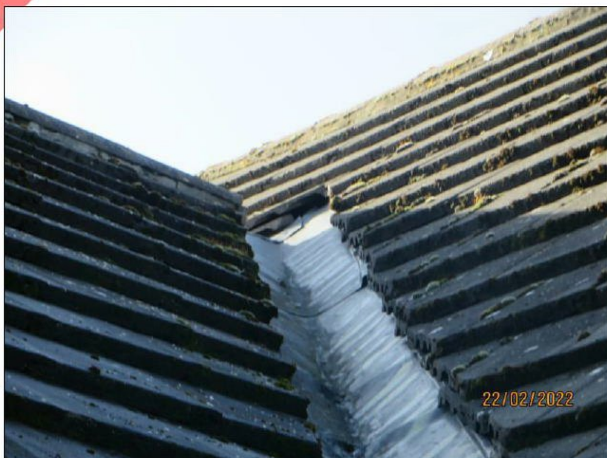
Figure 28. Gap present under roof tiles on outbuilding.
