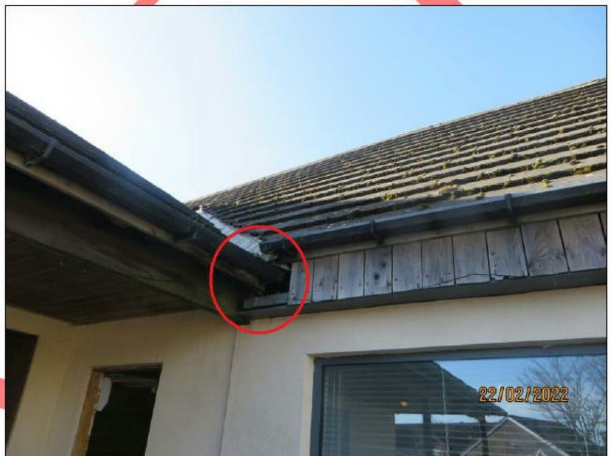
Figure 24. Gap present into wooden cladding on outbuilding.
