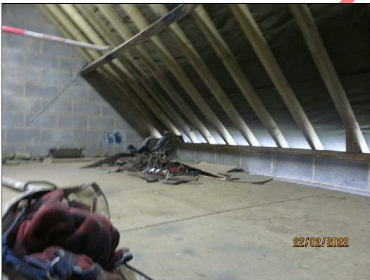
Figure 33. Storage area upper section where bat droppings found. Light ingress can be seen along wall tops.
