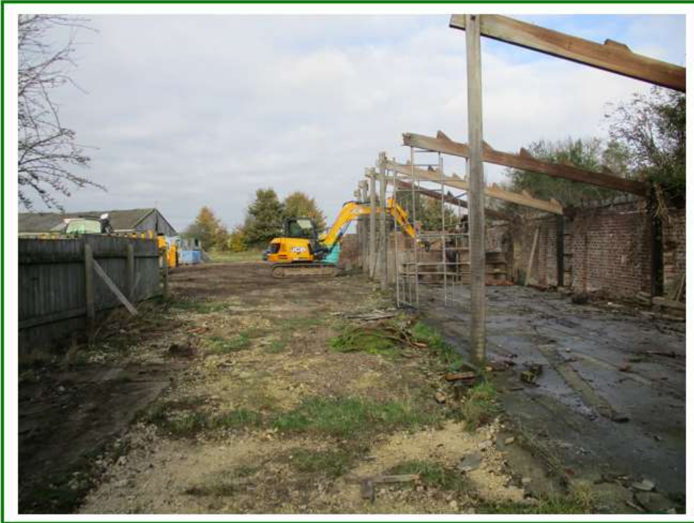
Photo No.4: Facing north showing demolished barn (right) and access to remainder of northern extent of site
