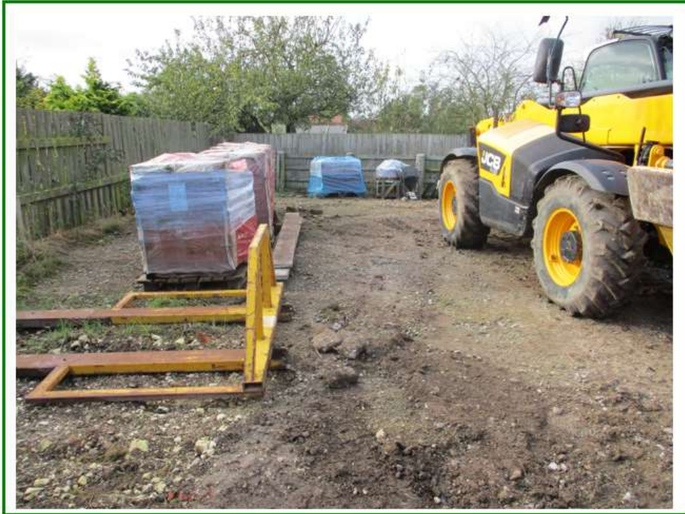
Photo No.6: Facing west from access track adjacent to demolished barn showing materials storage in west of site
