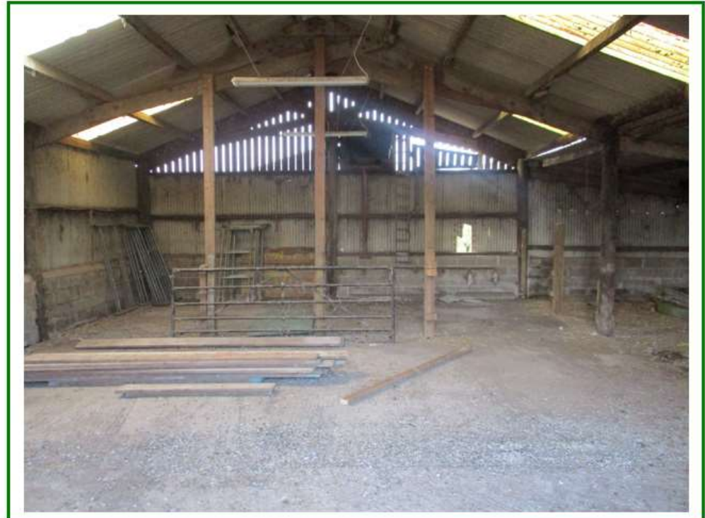
Photo No.10: Facing west showing interior of the barn and concrete flooring along with PACM composition of barn
