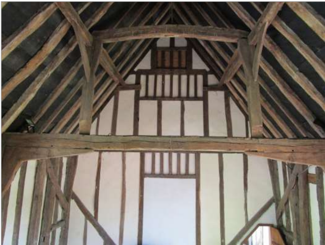
Fig. 35: Former barn interior, looking east from the gallery. The timber framing of the walls and the mullion windows are largely a twentieth century confection, although the tie beams and queen post roof are likely to be historic. Note the exposed roofing felt; there is currently no roof insulation.
