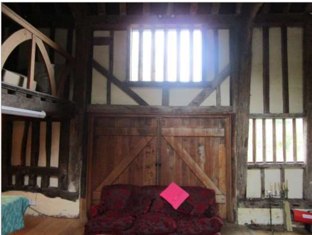
Fig. 41: The north wall of the former barn, showing the 1990s barn doors. These will be replaced like-for-like (on account of the floor lowering), and augmented by inner doors. To the left, a mullion window is proposed in the blocked door opening below the gallery.
