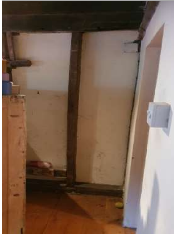
Fig. 38: A closer view of the wall shown in fig. 37, with the furniture removed. A single slender stud (not pegged into the sole plate or mid-rail and not original) will be removed in order to form an opening to the proposed larder. The sole plate will remain in situ.
