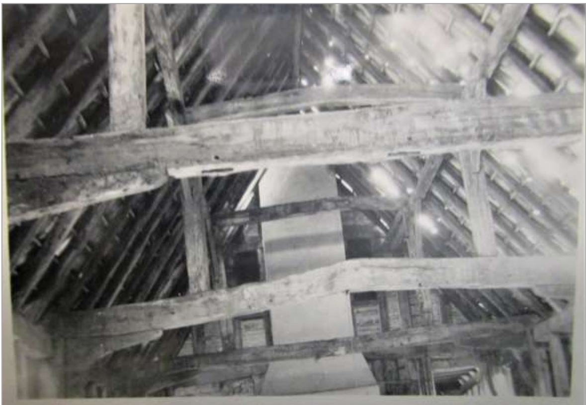
Fig. 11: Barn interior, looking south towards stack of former dairy, c.1965? (SPAB file)
