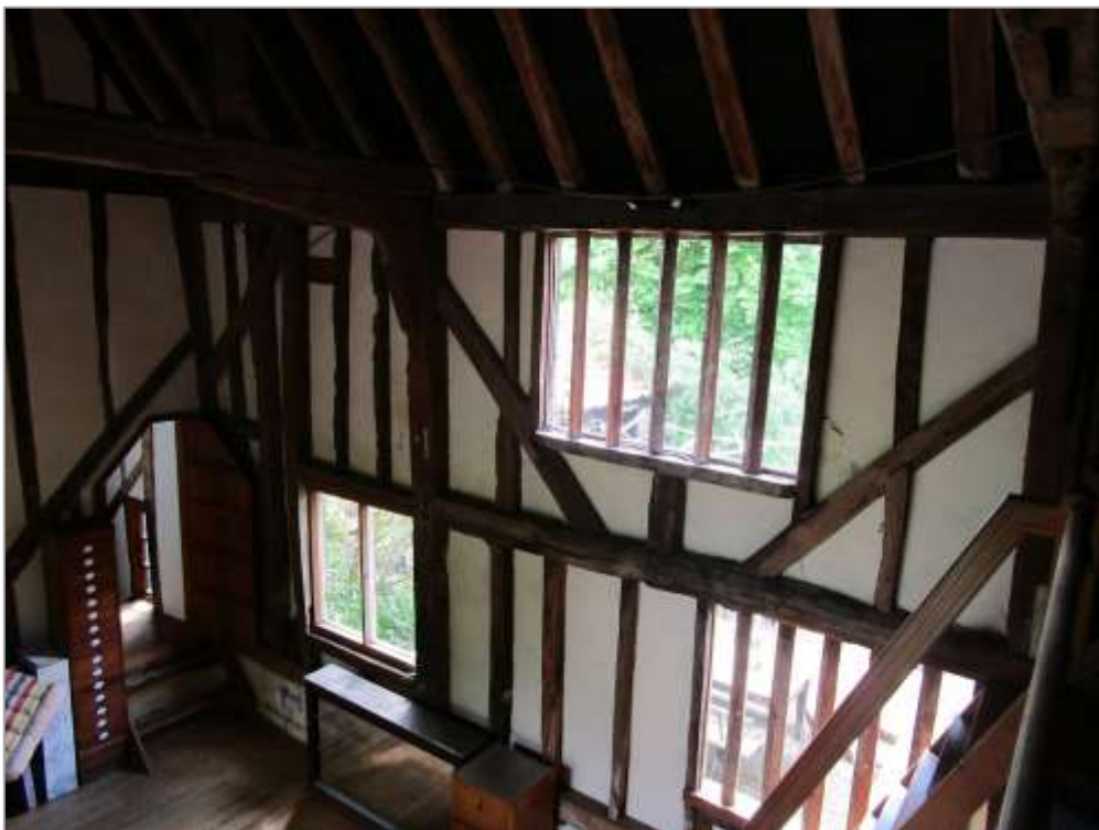
Fig. 39: The south wall of the former barn, viewed from the gallery. All the timbers of the central bay (between the two wall posts) are re-used and installed in the mid-twentieth century, when the brick plinth was also extended. It is proposed to form an opening below the mid-rail of this bay and reinstate barn doors, as shown on the c.1870 plan. Note also the 1979 ground floor window to left and the 1990s opening in the studwork of the east wall, connecting the barn to the accommodation in the eastern range.
