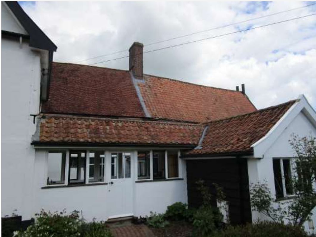
Fig. 34: The entrance lobby and link, built in 1993. This will be removed, and a new open-sided, gabled porch built in front of the present utility room (right).
