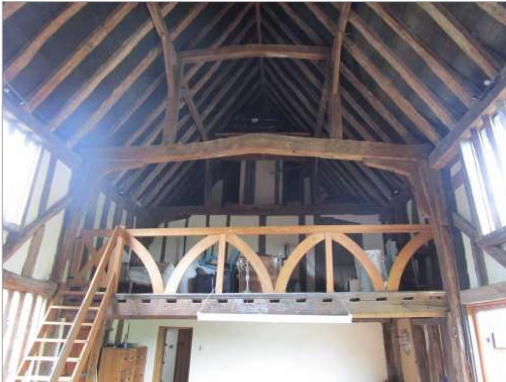
Fig. 36: Former barn interior looking west. There may historically have been an intermediate floor at this end, but the present gallery appears to be of mid-twentieth century date, re-using a chamfered beam (with mortices now on the vertical side). The gallery front and steep stair access date from the 1990s; they are hazardous and non-compliant with building regulations; the stair will be removed and more suitable balustrading provided in the gallery front. The gallery space will be an office area accessed from the bedroom beyond.
