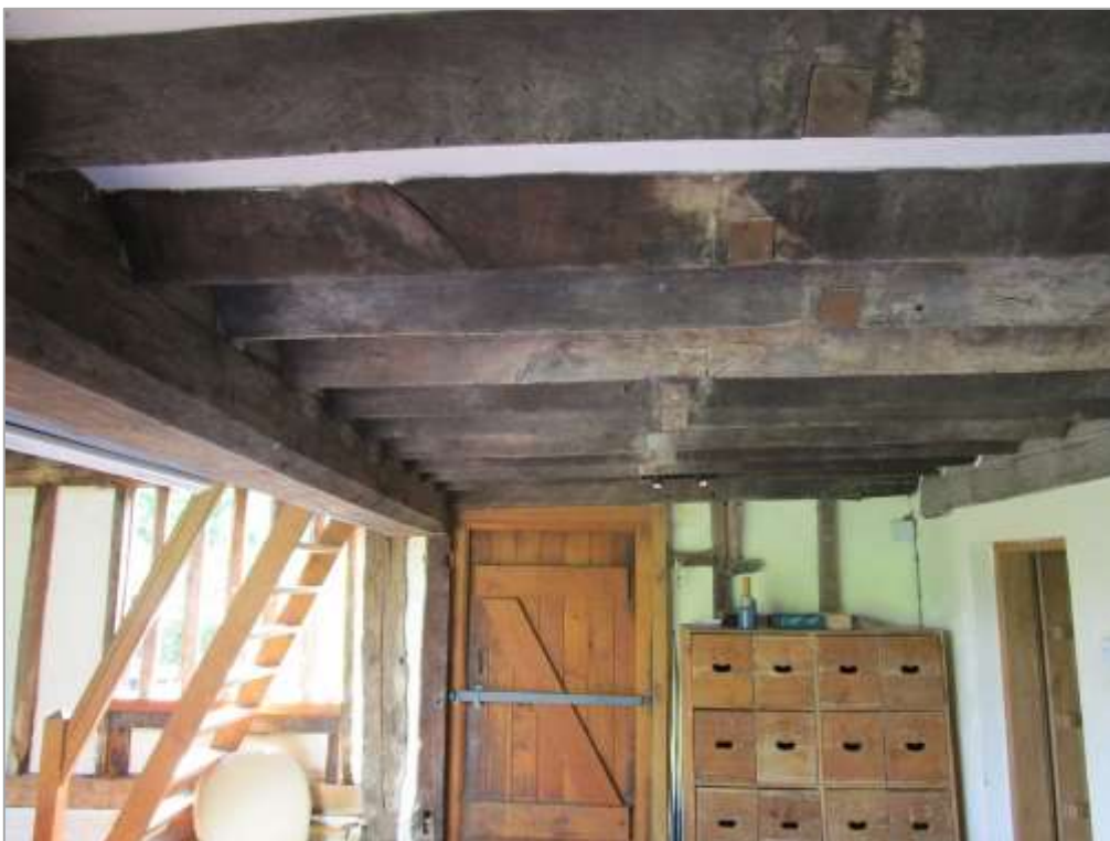
Fig. 37: The underside of the gallery has joists placed on the diagonal. Also shown here is the modern south door which will be removed under current proposals, with the opening blocked.
