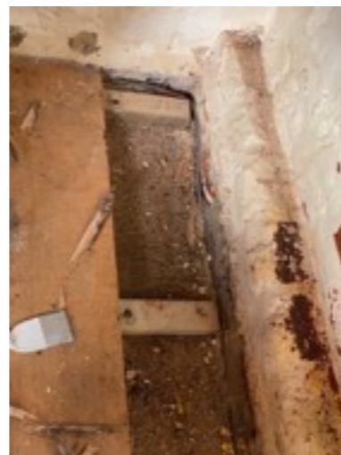
Existing concrete floor slab and edge of DPM, signs of paint blistering shows that excess moisture build up is present.
