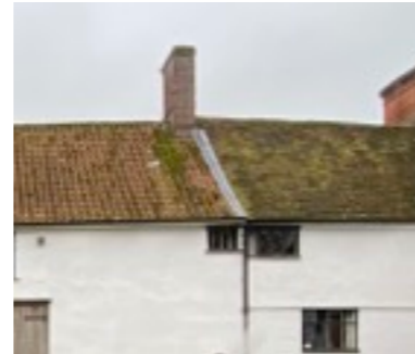
Messy lead flashing detail between the barn roof and main house.
