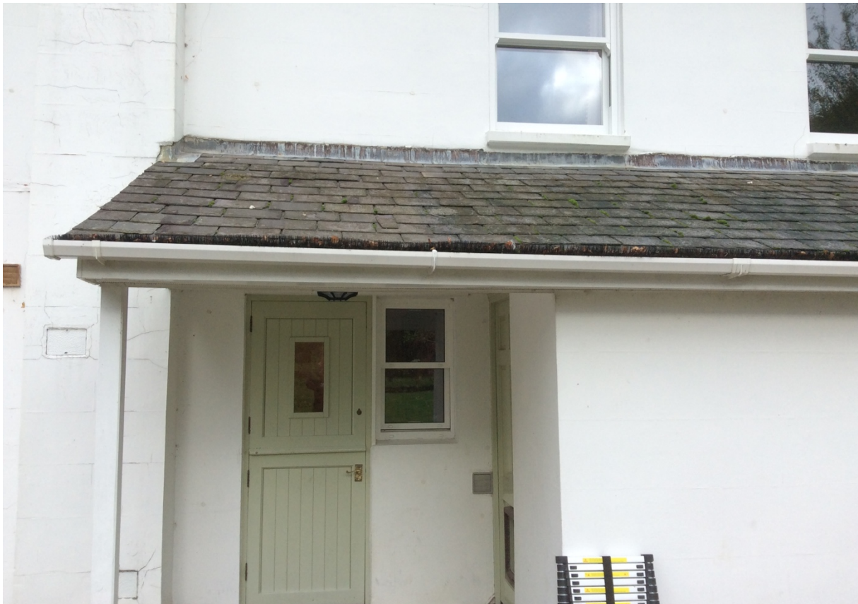
Figure 9. The slate roof tiles are mostly tight fitting with a maximum of 2 gaps with the potential to support bats.
