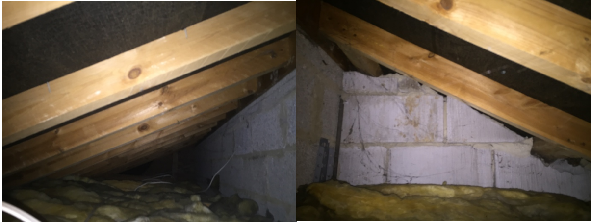
Figure 10. The small void of the single story sloped roof section which is low in height and has heavy cobwebbing.
