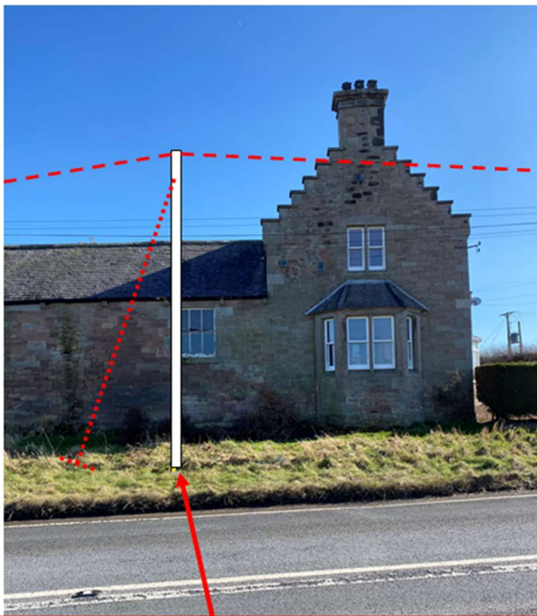
ERECT 1 x 9m MEDIUM POLE AND FIT STAY FOR ROAD CROSSING. LABEL AS CP1A. GRID REF. - 395336,649984 RENEW 2 SPANS OF 10/0.5 A/CABLE, 3 X D/W AND 1 X FIBRE CABLE FROM DP751 TO DP752 VIA NEW CP1A.
